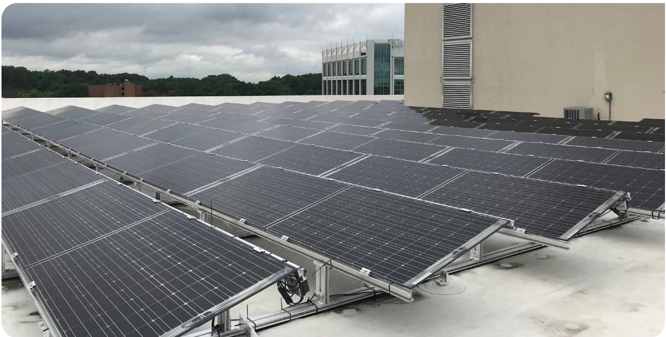
First solar energy system on a commercial property financed by Montgomery County's Commercial Property Assessed Clean Energy (C-PACE) financing program
