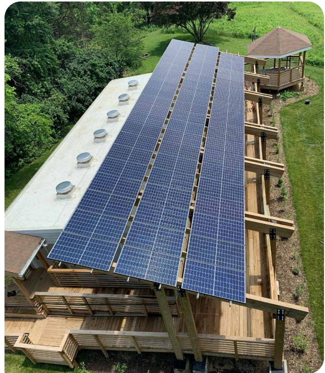
Solar array at M-NCPPC’s Maydale Conservation Park
