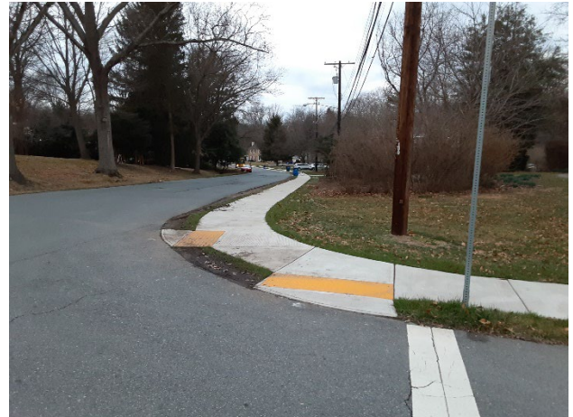
Figure 15 – New ramps with detectable warning surfaces installed as part of neighborhood sidewalk construction.
