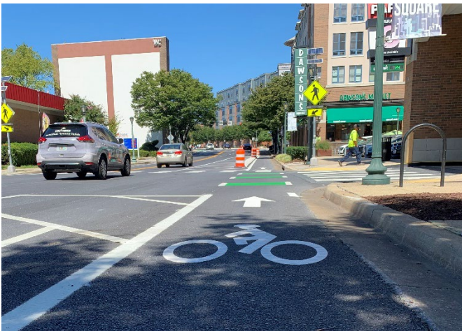
Figure 9 - City of Rockville installing protected bike lane along North Washington Street summer 2023.
