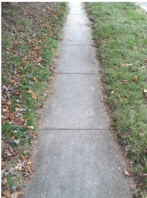
Figure 2 – Example of Non-Compliant Sidewalk
