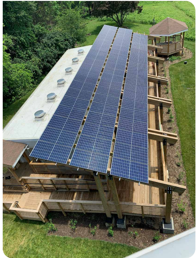
Solar array at M-NCPPC’s Maydale Conservation Park
