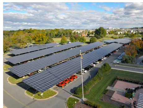
Microgrid at the Public Safety Headquarters
