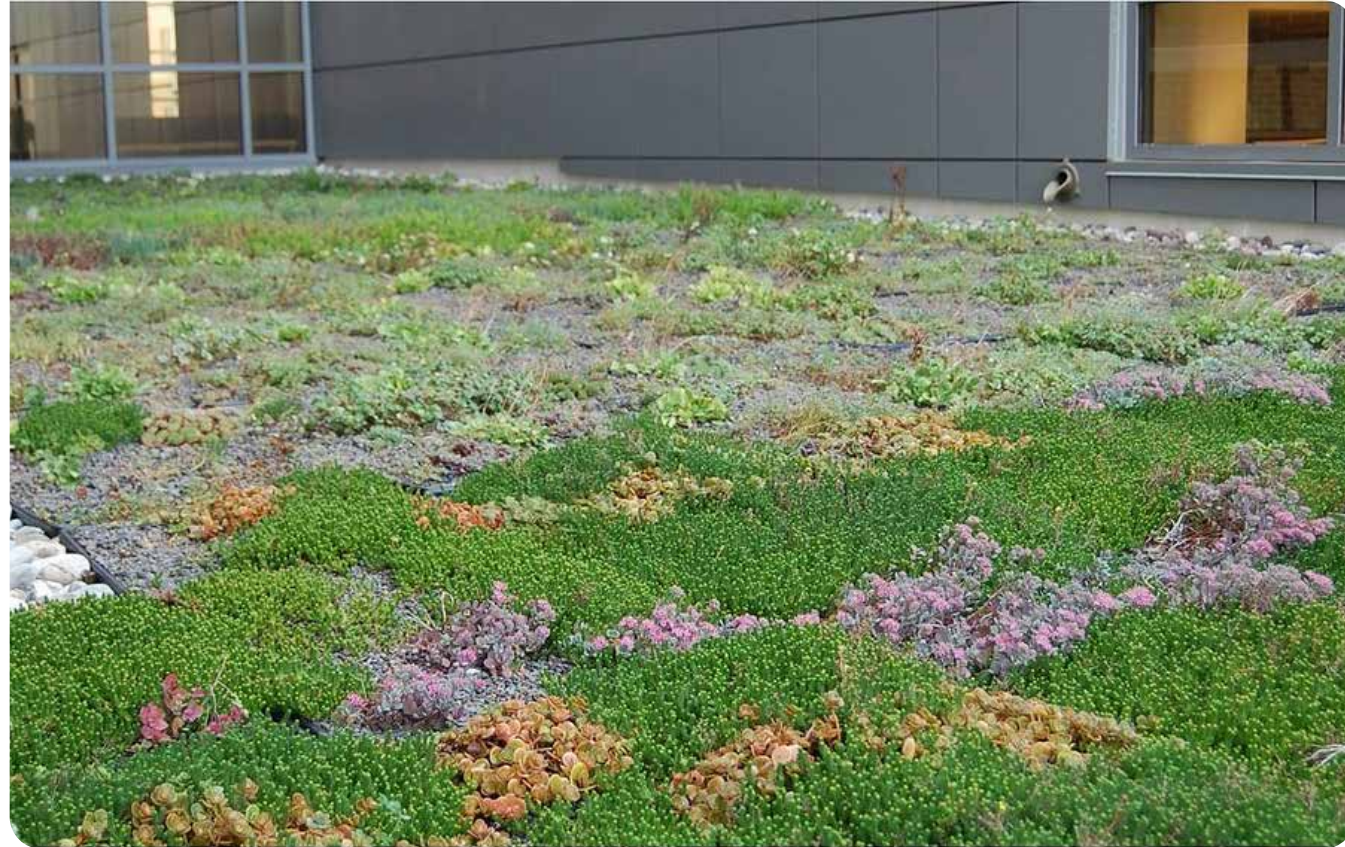
Among other benefits, green roofs reduce urban heat island effect and increase urban greening
