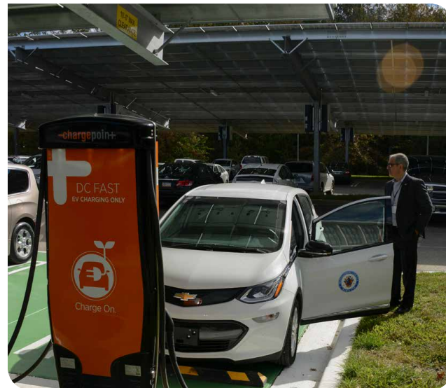
Charging a Montgomery County electric vehicle
