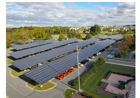
Microgrid at the Public Safety Headquarters
