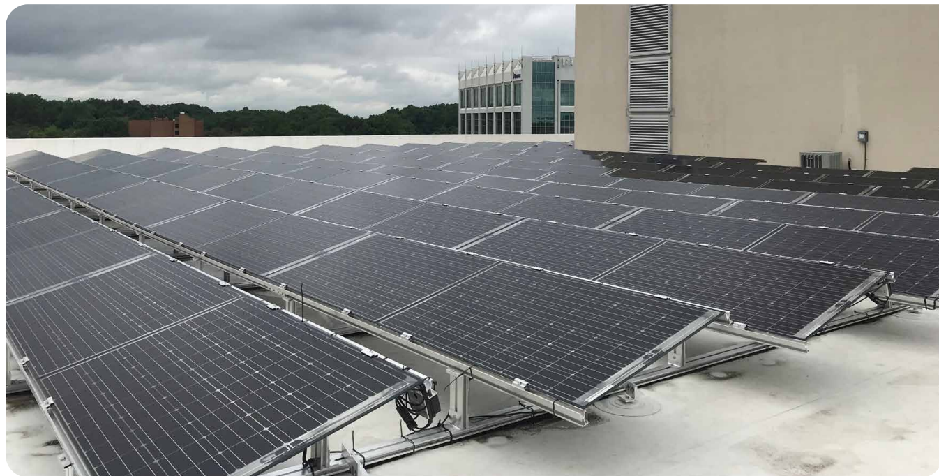
First solar energy system on a commercial property financed by Montgomery County’s Commercial Property Assessed Clean Energy (C-PACE) financing program
