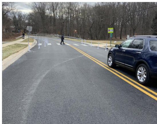
Example of using flex posts to shorten crossing distances for people walking and biking where Sligo Creek Trail crosses Dennis Avenue.
