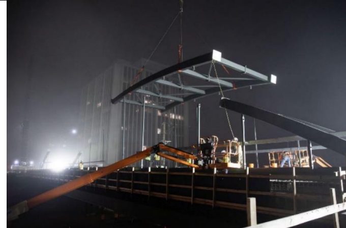
New pedestrian bridge installed over Connecticut Ave for the future Purple Line and Capital Crescent Trail.
