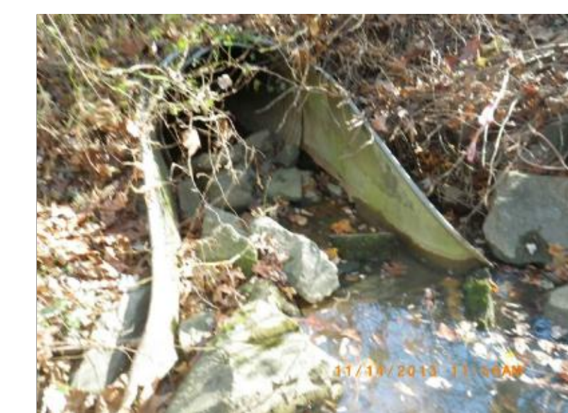
FIGURE 3. UPGRADE RIPRAP CHANNEL AT POND OUTFALL TO REDUCE DISCHARGE VELOCITIES TO NON-EROSIVE LEVELS.
