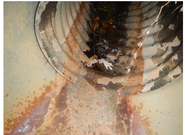
[Photo 1] Existing Eroded CMP Outfall Pipe
