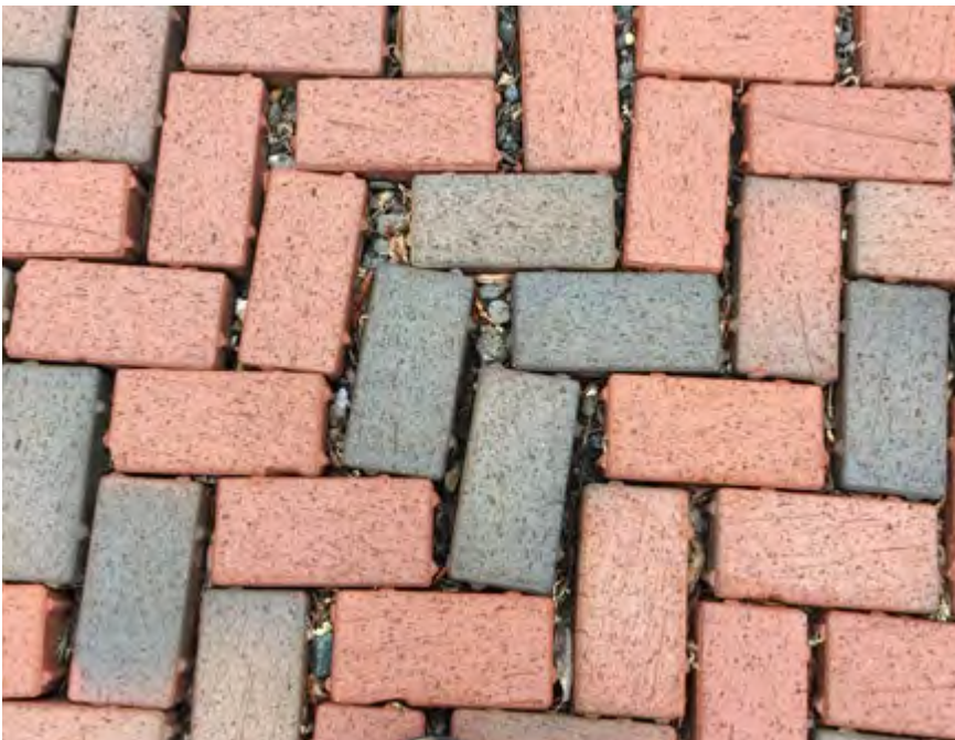
Poorly aligned pavers
