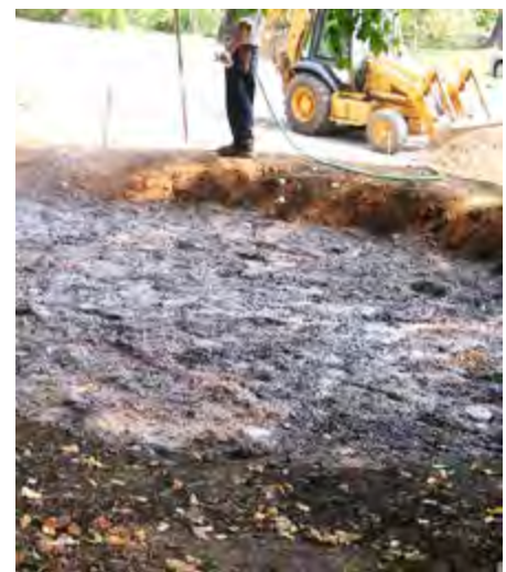
Planting media is installed. Final media elevation is 6" below berm top or weir notch elevation if using a weir.
