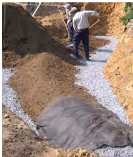
Pipe is covered with 57 stone gravel, then a layer of geotextile before placing the planting media.
