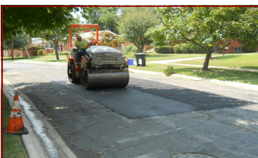
Distressed areas will be patched prior to resurfacing
