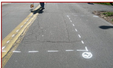
Typical patching paint markings
