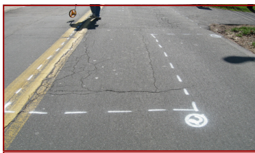
Typical paint markings
