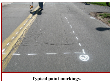
Typical paint markings.
