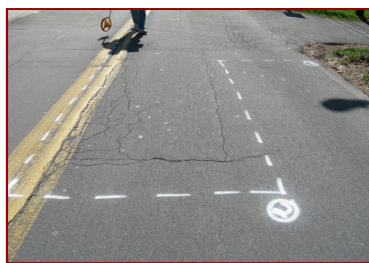
Typical paint markings.
