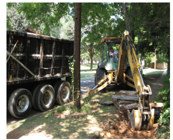
Defective concrete is removed
