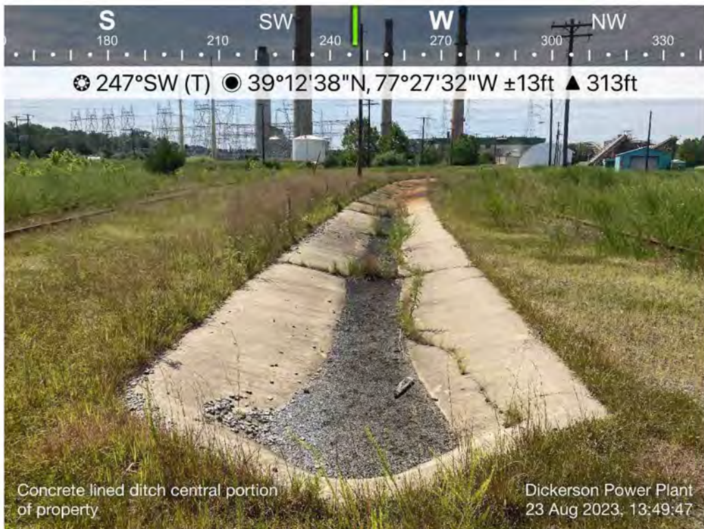
22. View of typical concrete-lined ditch in the central portion of the site (08/23/23).
