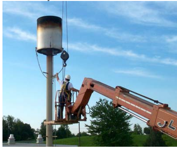
Maintenance Being Performed On The Gas Flare System at The Oaks Landfill
