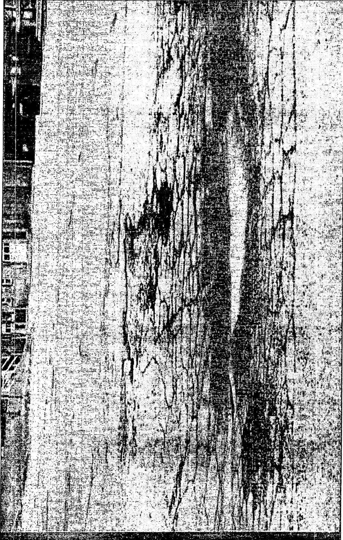
Seven Locks Road Parking Lot – Repairs Needed
