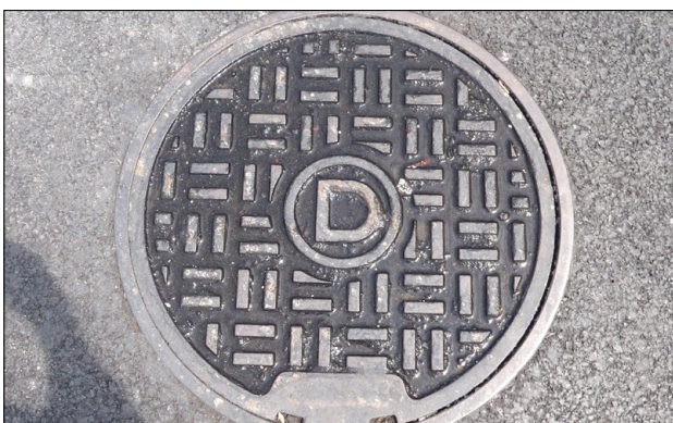
Flow splitter manhole cover
