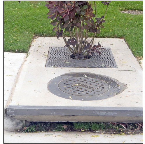
Vegetation and debris clogging the inlet, as shown here, should be removed.
