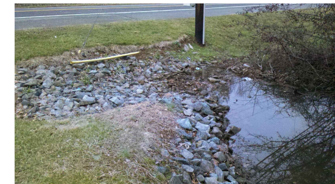
FIGURE 1. EXISTING EROSION TO BE REPAIRED AND OUTFALL DESIGNED TO MINIMIZE FUTURE EROSION.
