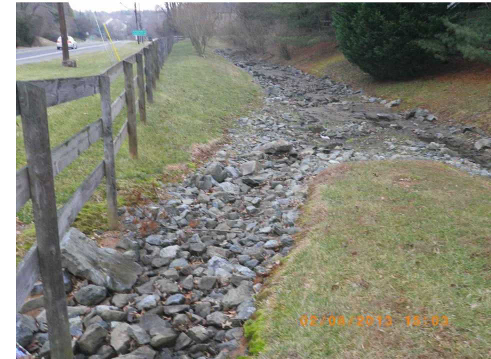
FIGURE 3. EXISTING UPSTREAM END OF FACILITY TO BE CONVERTED TO INFILTRATION AREA TO INFILTRATE STORM WATER. TREE SCREENING TO REMAIN.
