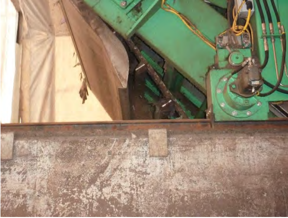
Photo 6 - Capacity Optimization Gate (COG) in closed position near bay discharge
