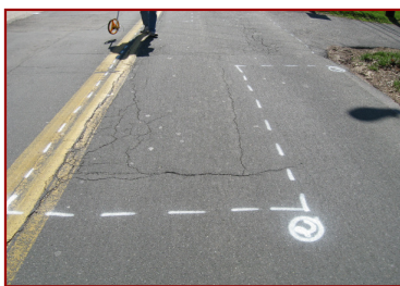
Typical paint markings.
