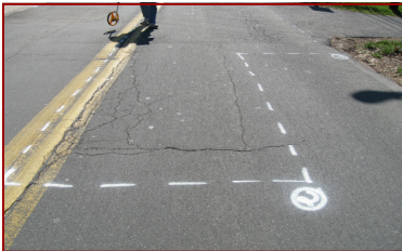
Paint markings outline areas to be patched.
