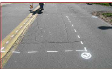
Typical patching paint markings
