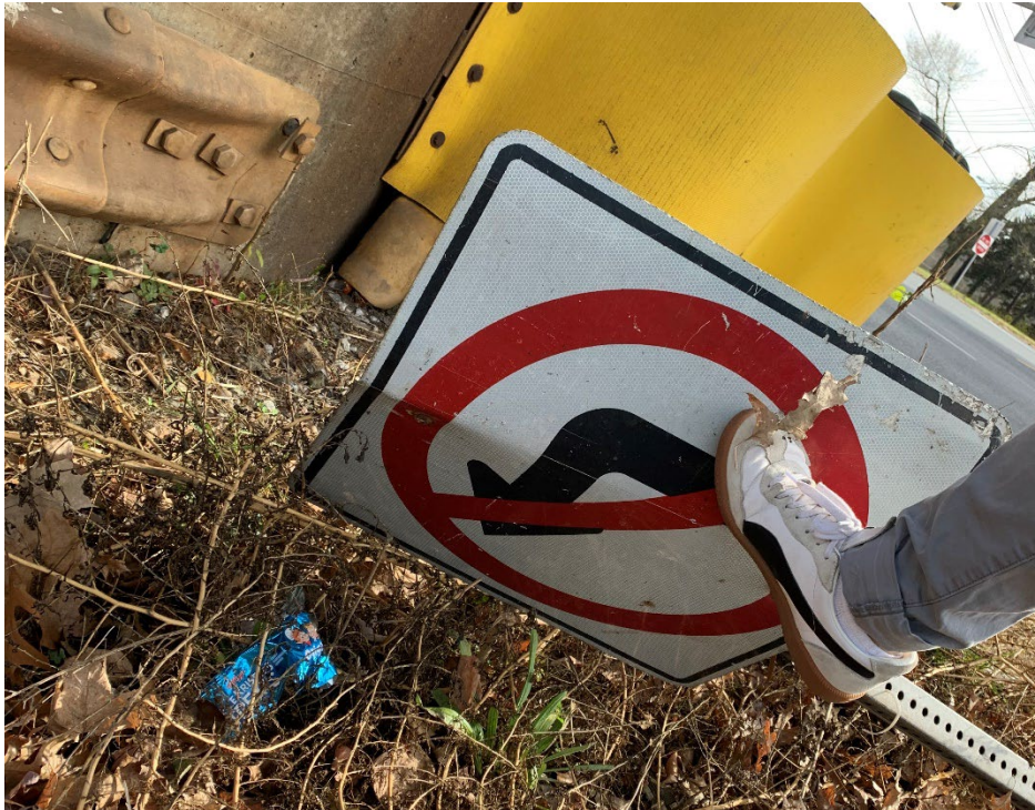
Picture 19: “No Left Turn” sign knocked-over and damaged at north leg median.
