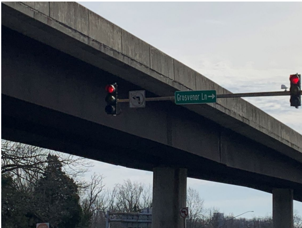
Picture 14: Faded “No Left Turn” sign on signal mast arm.
