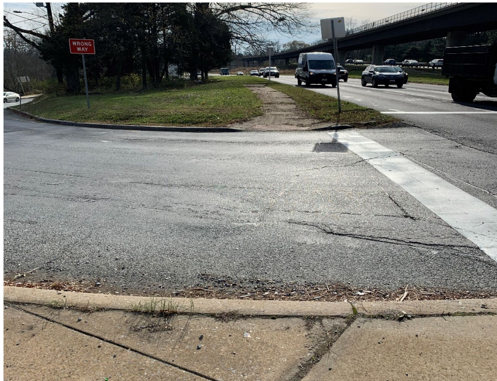
Picture 8: No ADA ramp/path across intersection to reach bus stop at SE corner of the intersection.
