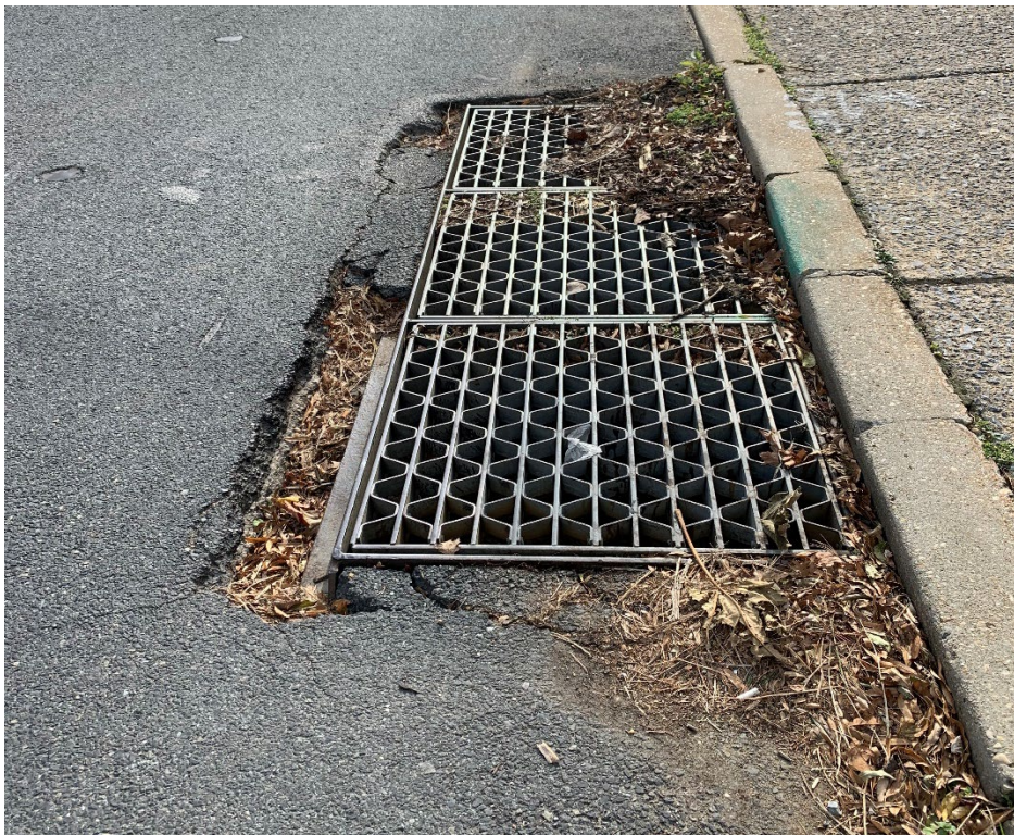
Picture 20: Debris, sediment build-up, and deteriorating pavement around grate inlet at the NW corner.
