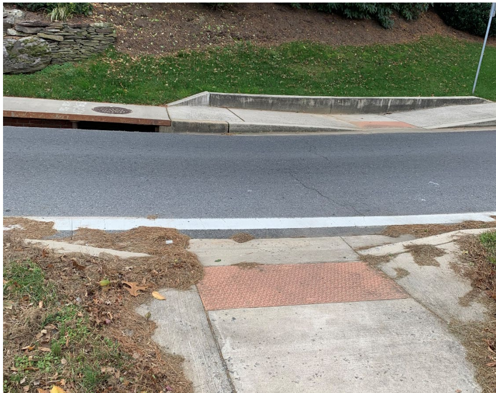
Picture 18: Unaligned ramps with screwed crosswalk at west leg slip lane.
