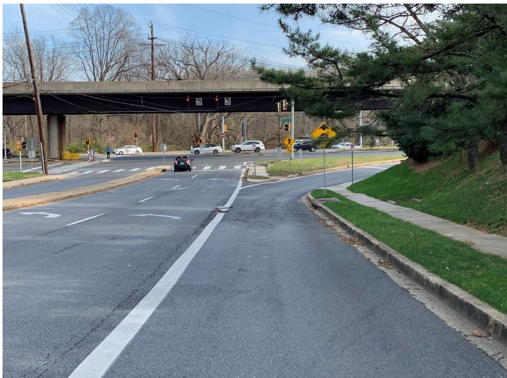
Picture 16: Tree branches blocks “Stop Ahead” sign. Cracked and fading left turn arrow pavement markings along west leg approach.
