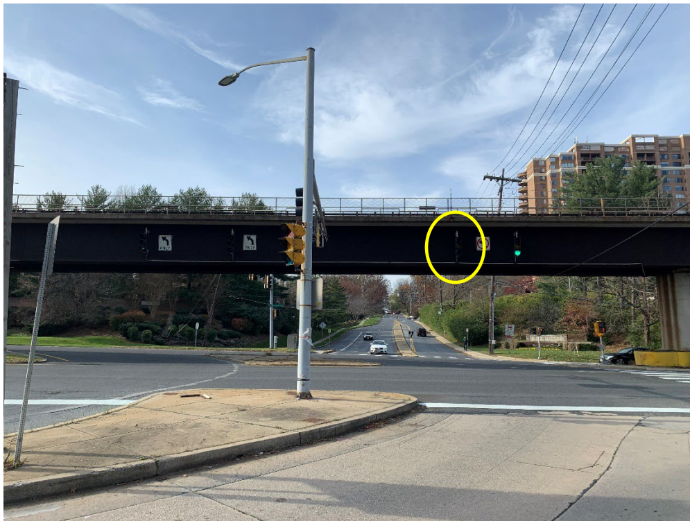
Picture 6: Signals facing east leg traffic. Green signal is out for through movement (see yellow highlight).
