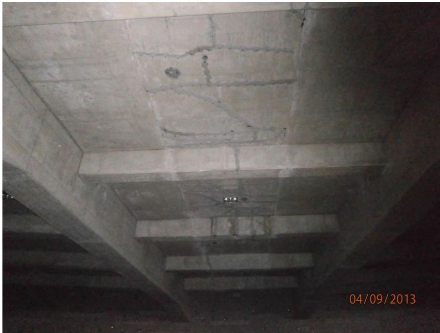
Image 7: Cracking Evident on Underside of Level 330 East Pour Strip – April 9, 2013
