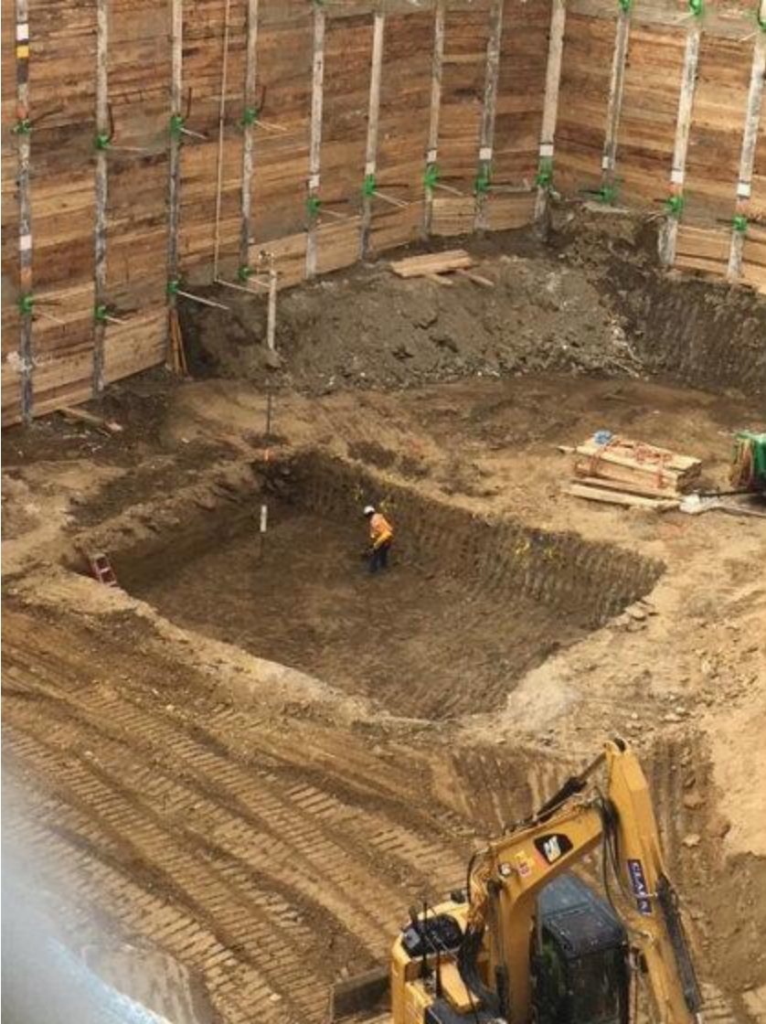
Footer for South Tower Crane
