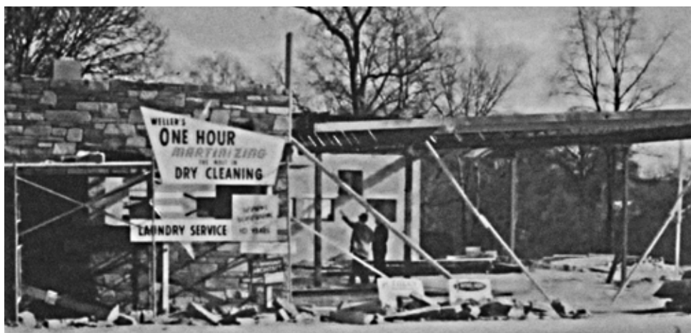
View of the Weller's Dry Cleaning under construction, c. 1961. Note the sign that reads "Weller's One Hour Martinizing The Most in Dry Cleaning." Source: Courtesy of Rose Jean Weller/Silver Spring Historical Society.
