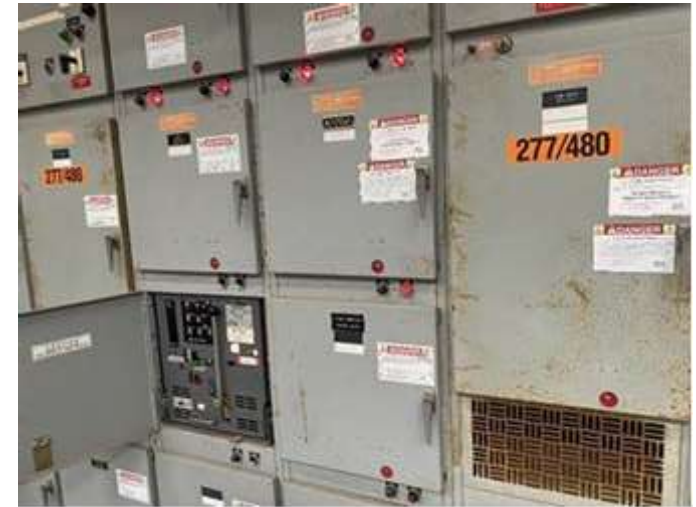
Potomac WFP Pump Station 2
