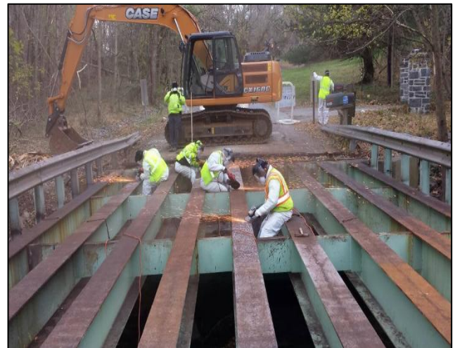
Highway Services Depot Crews replace the bridge deck span along Huntmaster Road in Damascus
