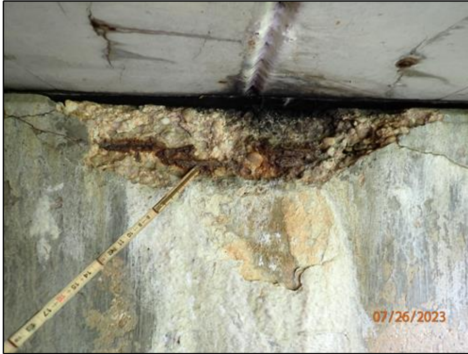
21. Spall with exposed and corroded reinforcement in the west abutment below Beams 14 and 15 (looking west)
