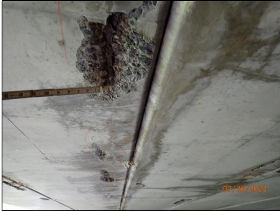
19. Spalls with exposed reinforcement along the south edge of Beam 14 near midspan (looking east)
