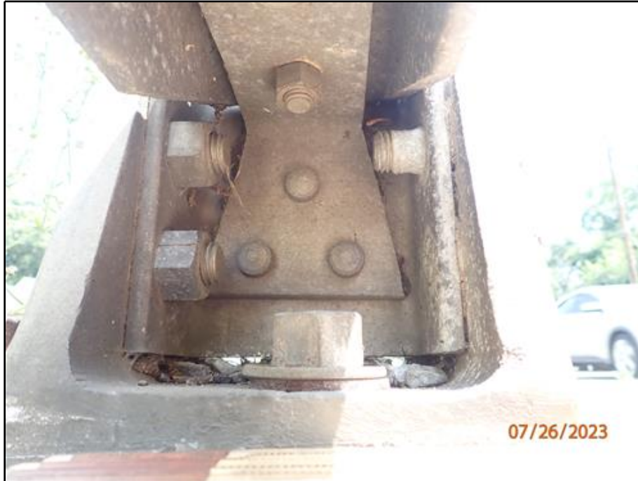
9. Sheared bolt, cracked and missing nut at Post 5 of the north railing (looking east)
