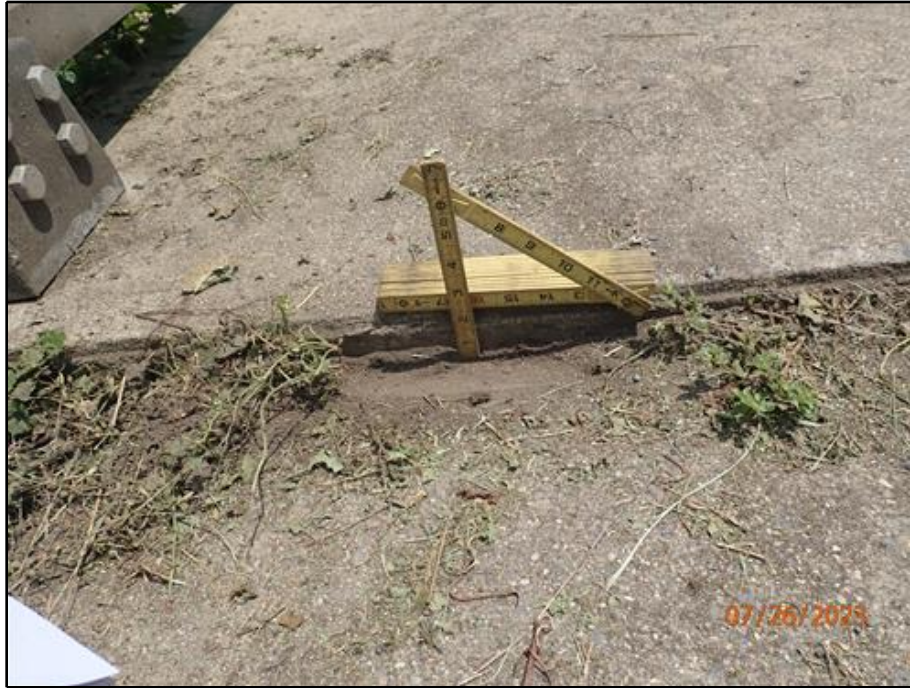
7. Vertical differential of the north sidewalk at the west end (looking east)
