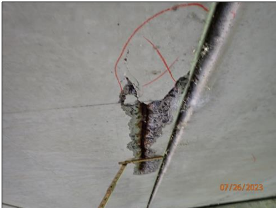
14. Spall with exposed reinforcement along the north edge of Beam 5 near the west abutment (looking west)
