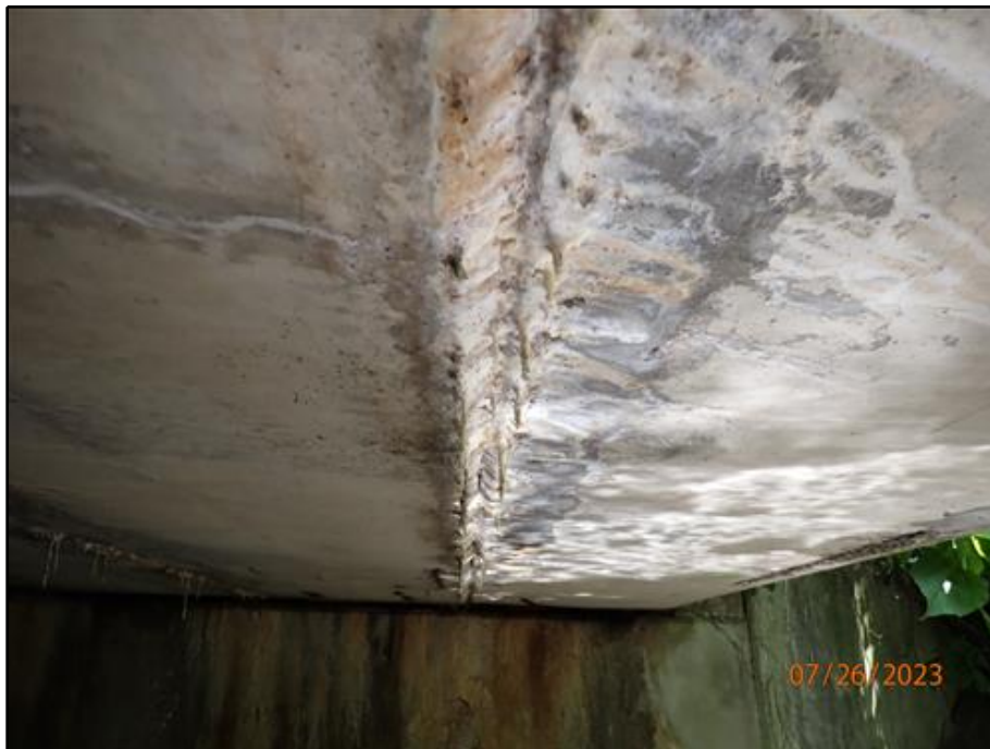
12. Water leakage and efflorescence between Beams 1 and 2 (looking east)
