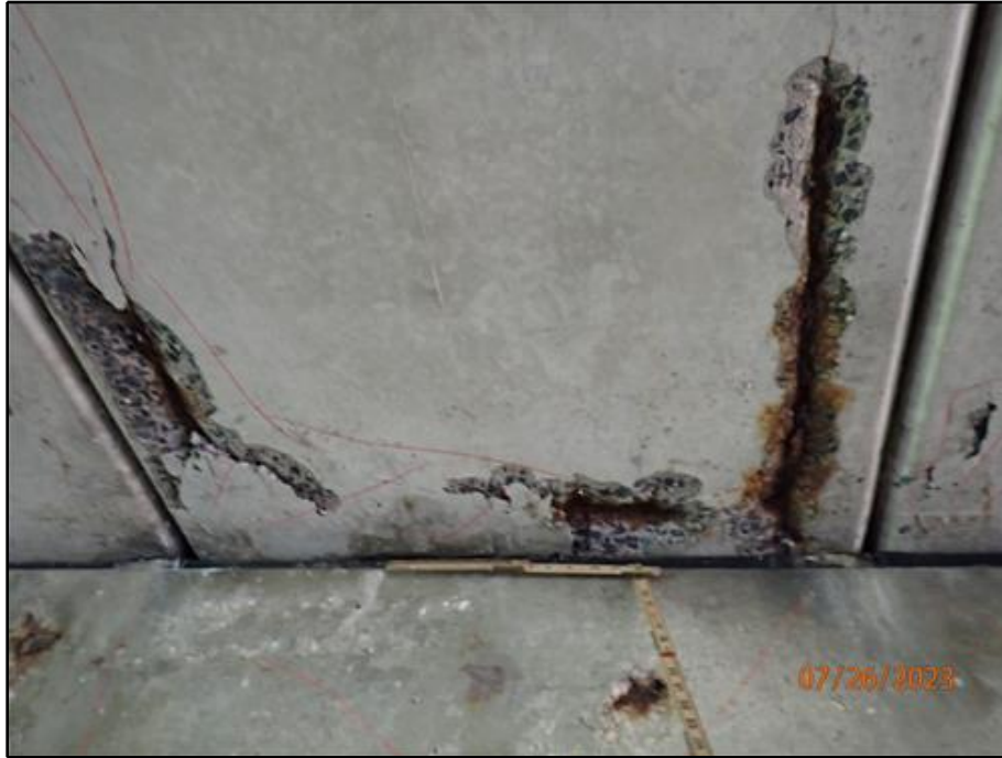
15. Delamination and spalling with exposed corroded reinforcement at the end of Beam 6 near the east abutment (looking east)
