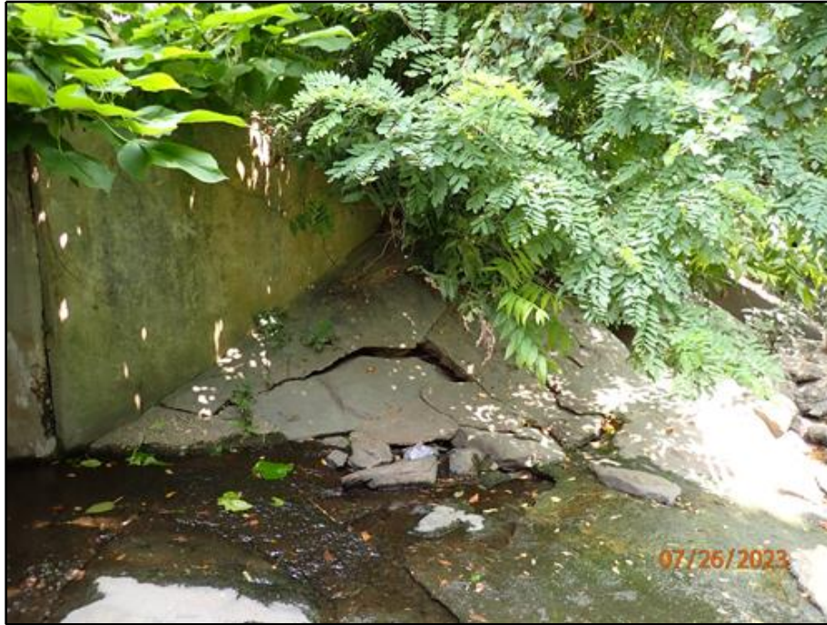
23. Fractured channel protection along the southeast embankment (looking east)
