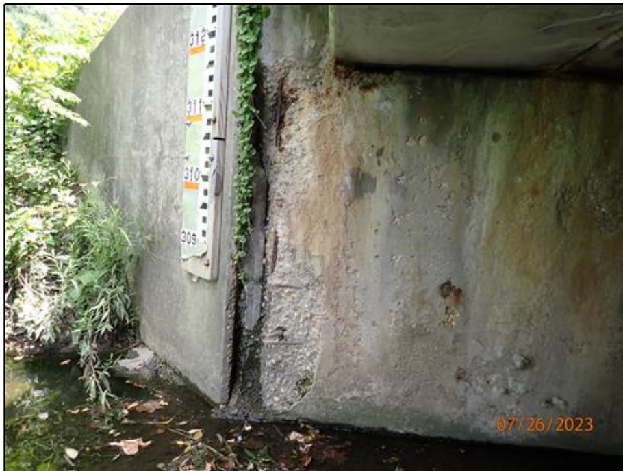
20. Spall with exposed reinforcement in the east abutment at the interface with the northeast wing wall (looking east)
