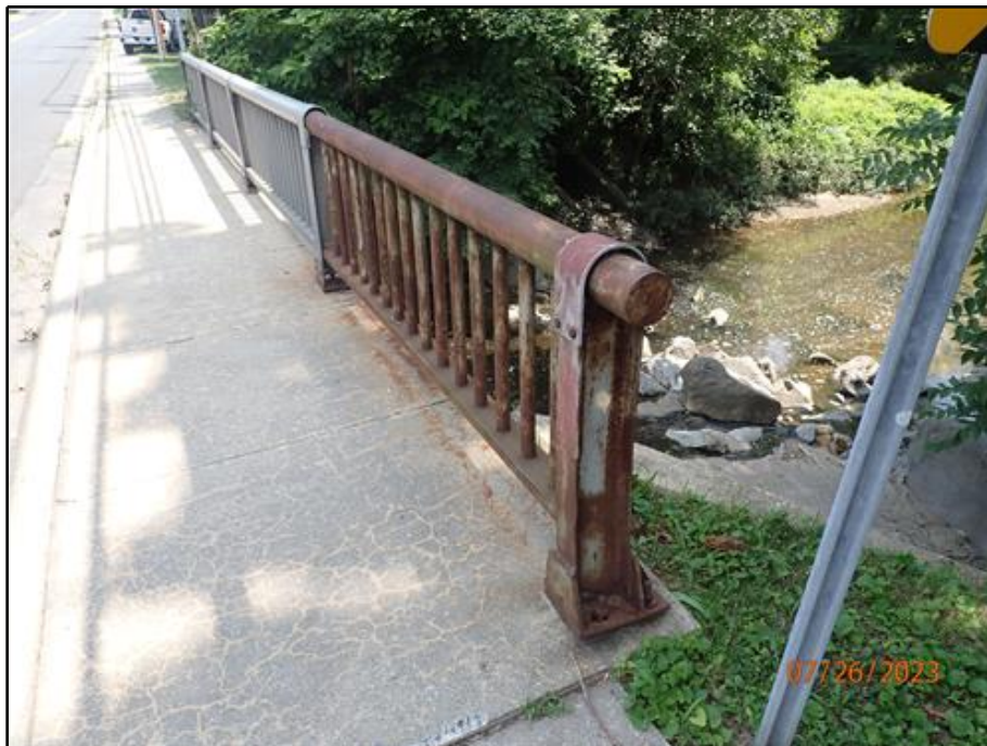
10. Moderate corrosion at the west section of the south railing (looking east)
