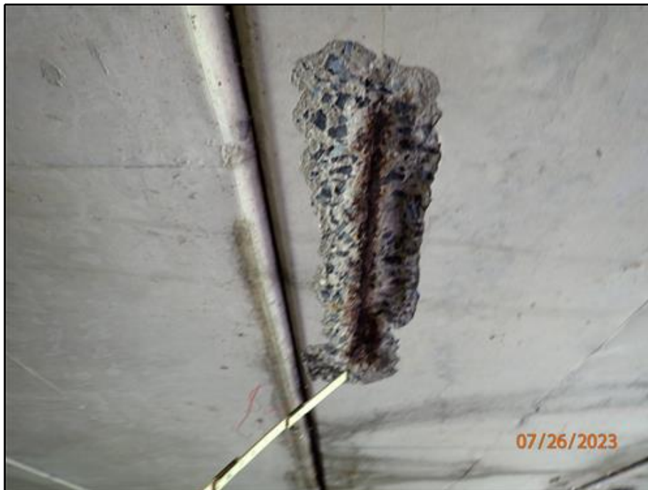
18. Spall with exposed reinforcement along the south edge of Beam 13 near midspan (looking west)
