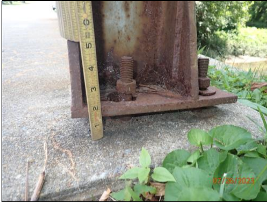
11. West baseplate of the south railing is lifted up (looking east)
