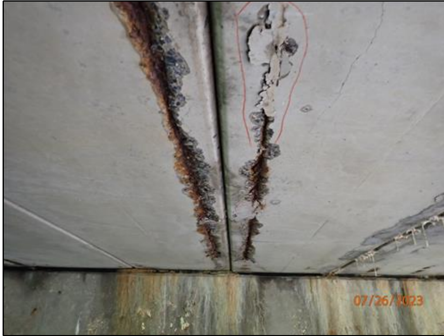
13. Spall with exposed reinforcement along Beams 3 and 4 near the east abutment (looking east)
