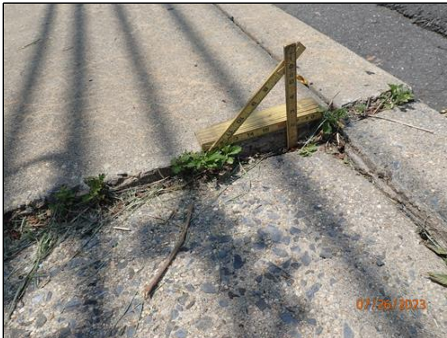
8. Vertical differential on the south sidewalk at the east end (looking west)
