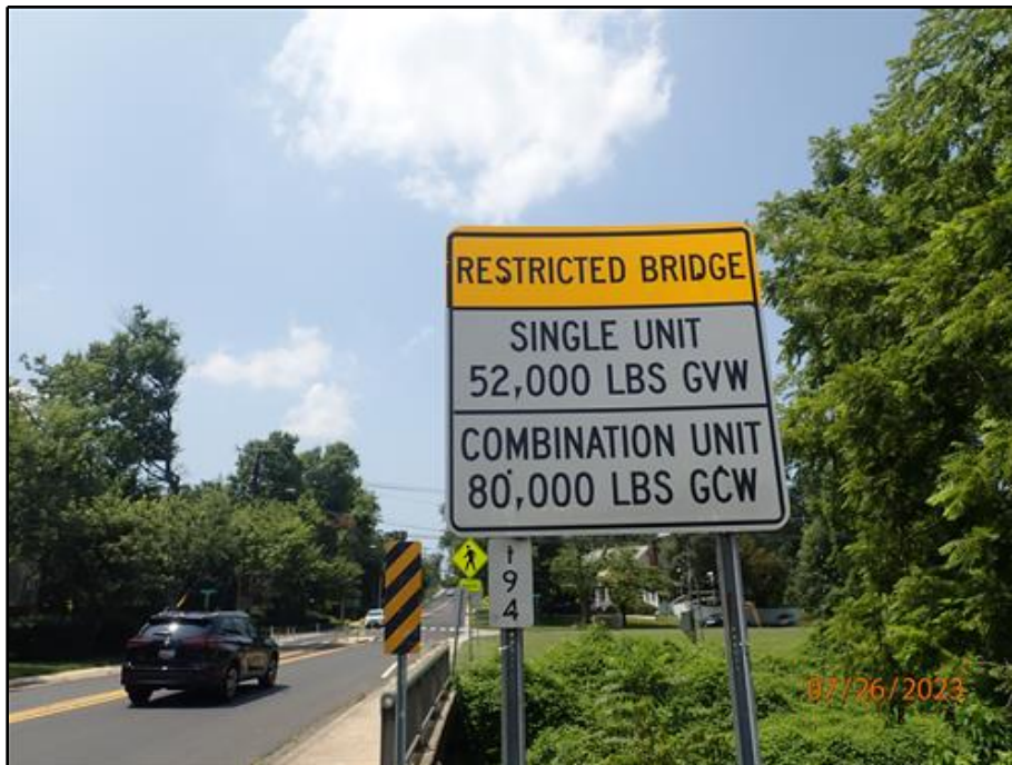
24. Load posting sign at the east approach (looking west)
