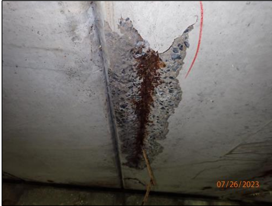
17. Spall/delamination with exposed reinforcement at Beam 9 starting at the east abutment (looking east)
