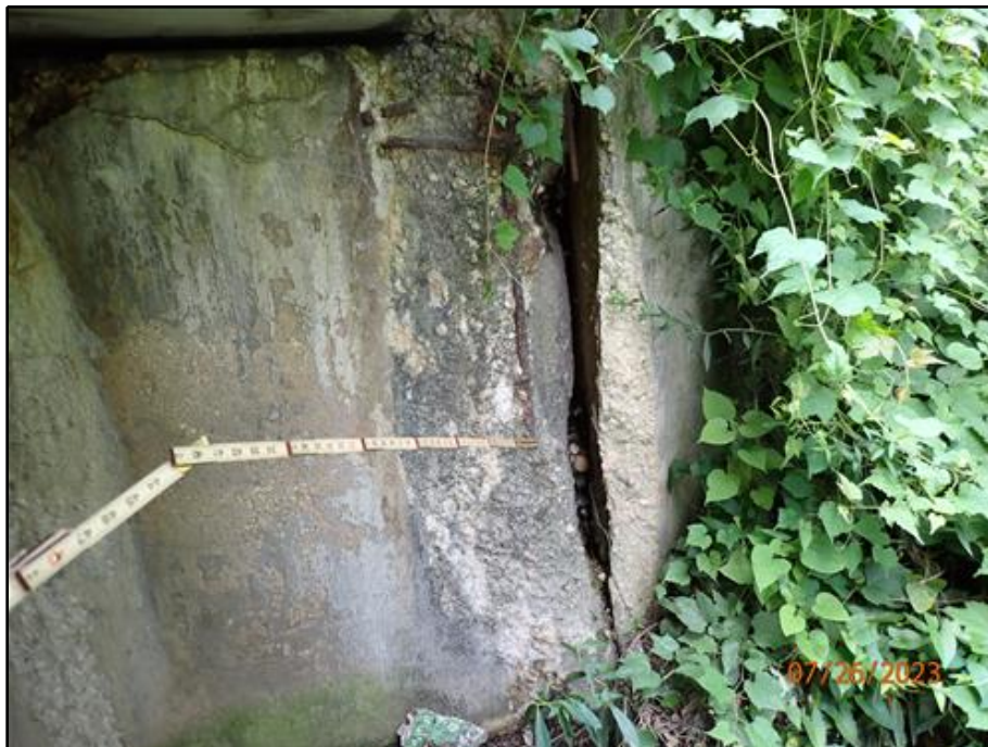
22. Spall with exposed reinforcement and fill infiltration in the west abutment at the interface with the northwest wing wall (looking west)
