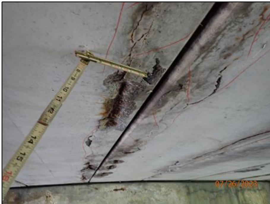
16. Spalls with exposed reinforcement at Beams 7 and 8 near mid-span (looking east)
