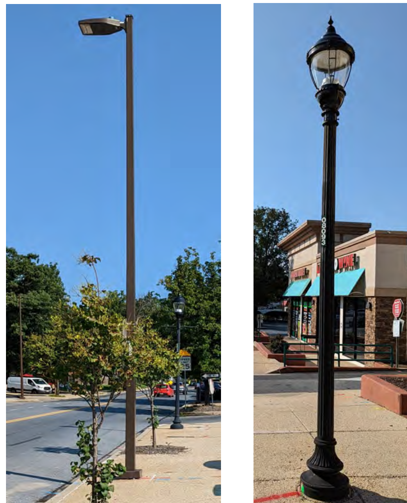
Figure 30 – Rectangular Light on pendent poles (left) and Washington Globe pedestrian light poles (right).
