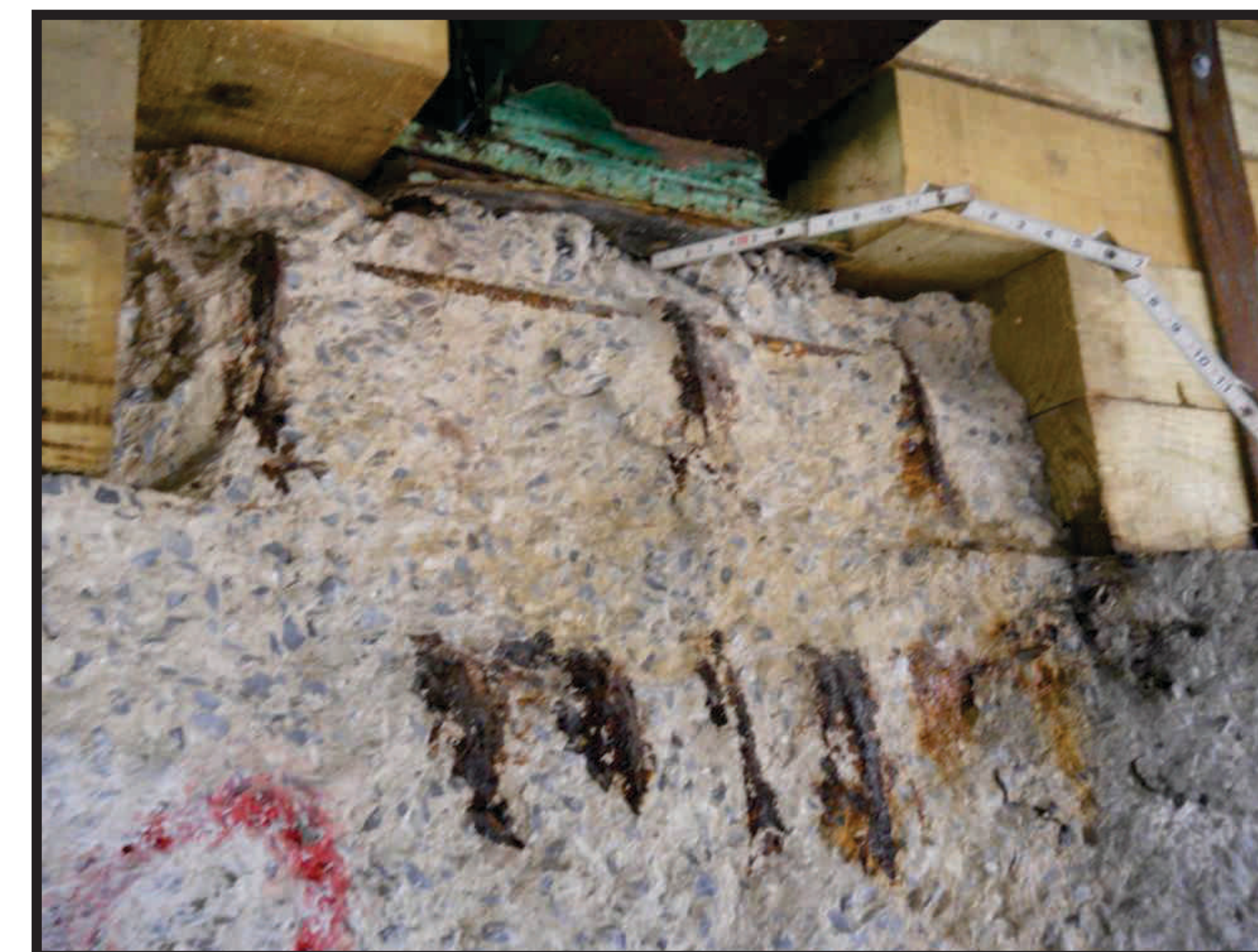
Pier bearing pedestal spalls
