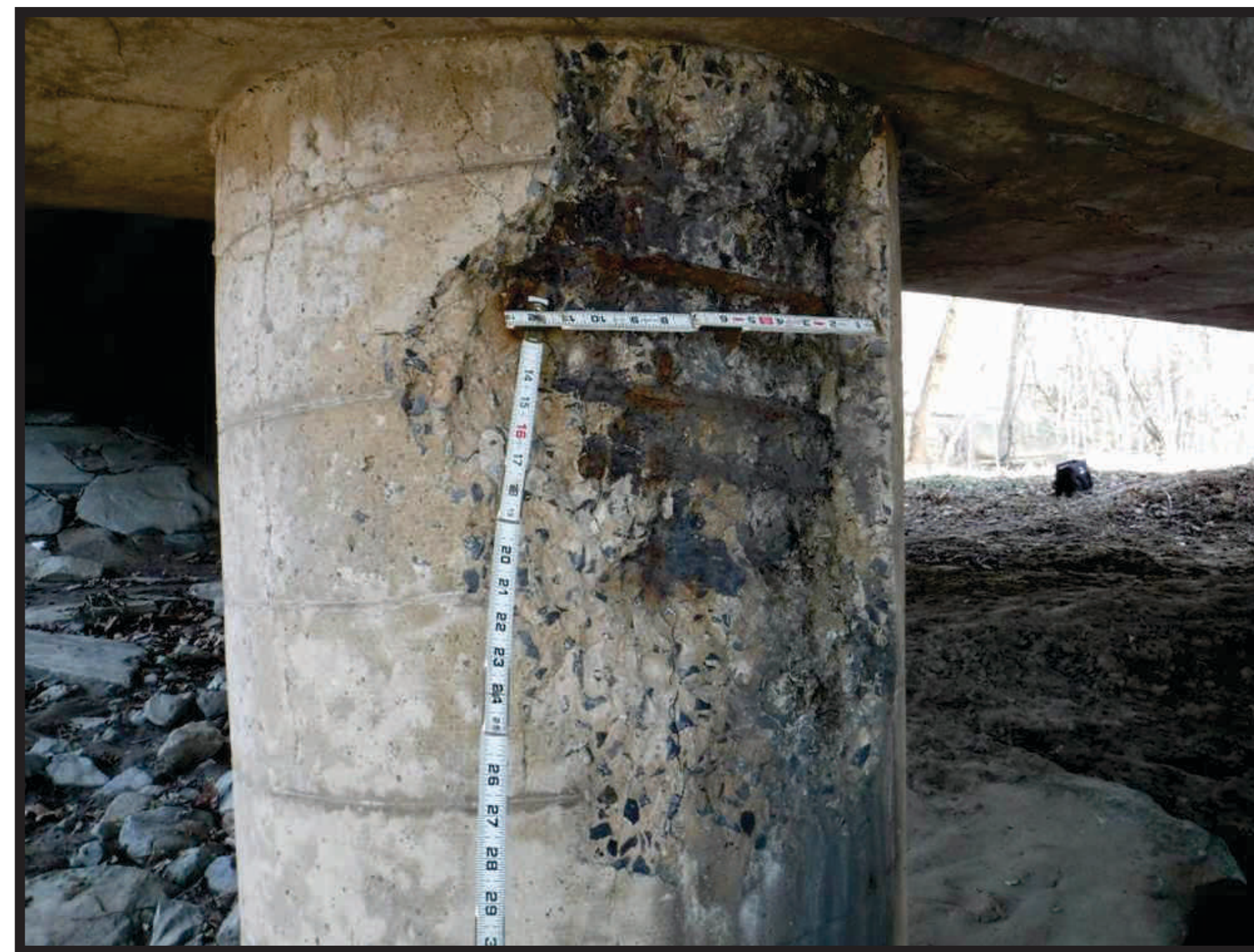
Pier column spalling
