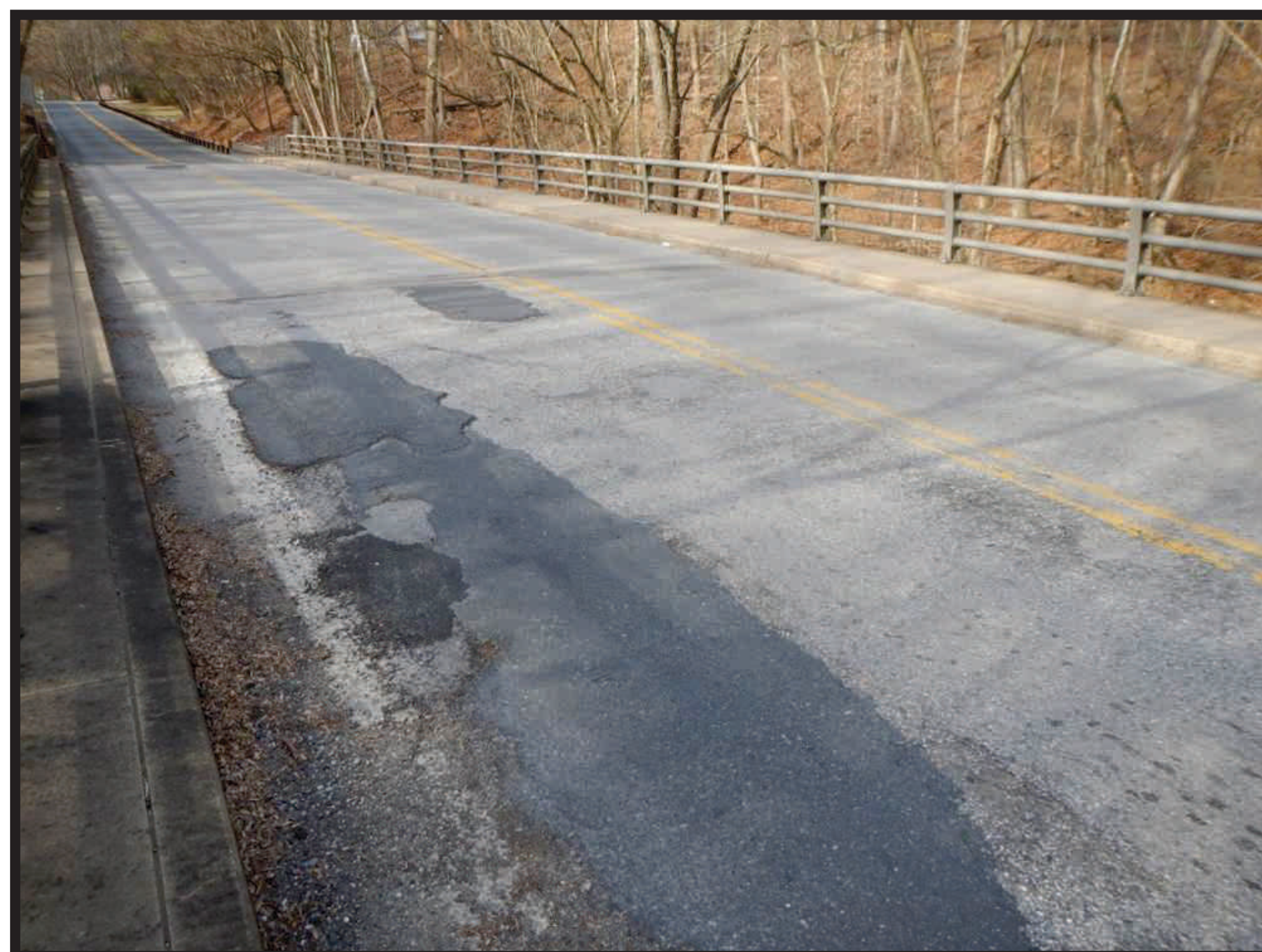
Wearing surface spalls and patching
