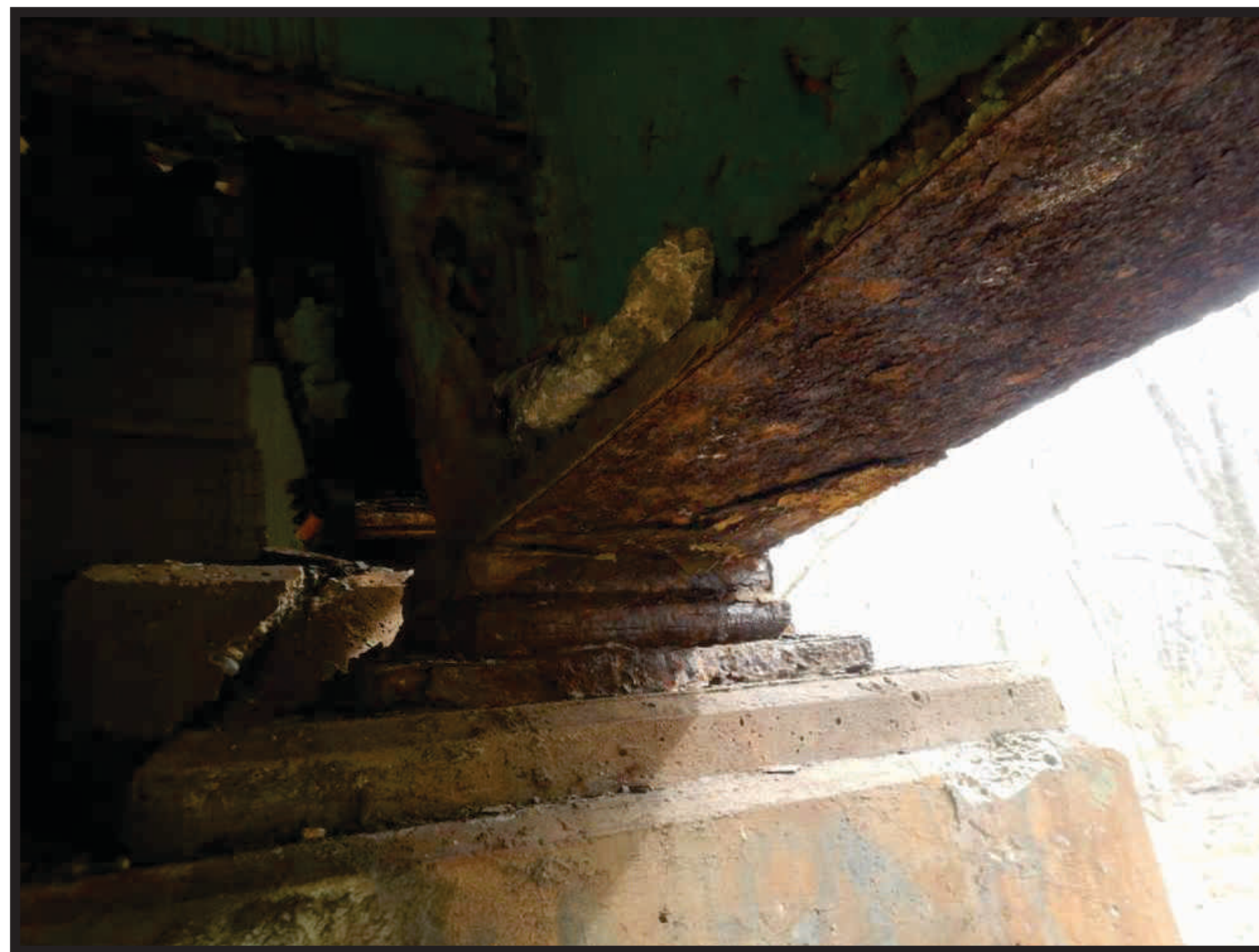
Steel corrosion and delamination
