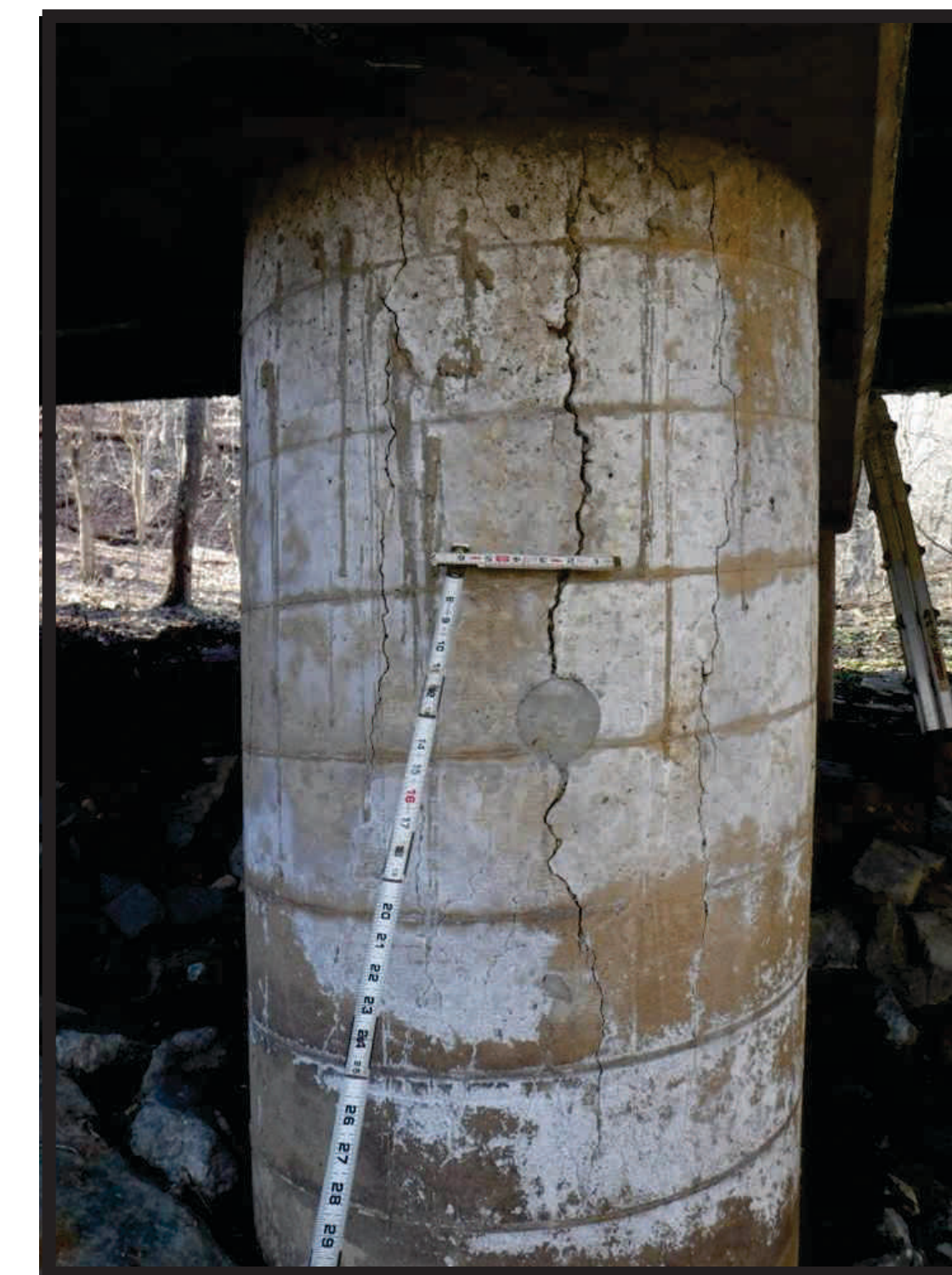
Pier column cracking
