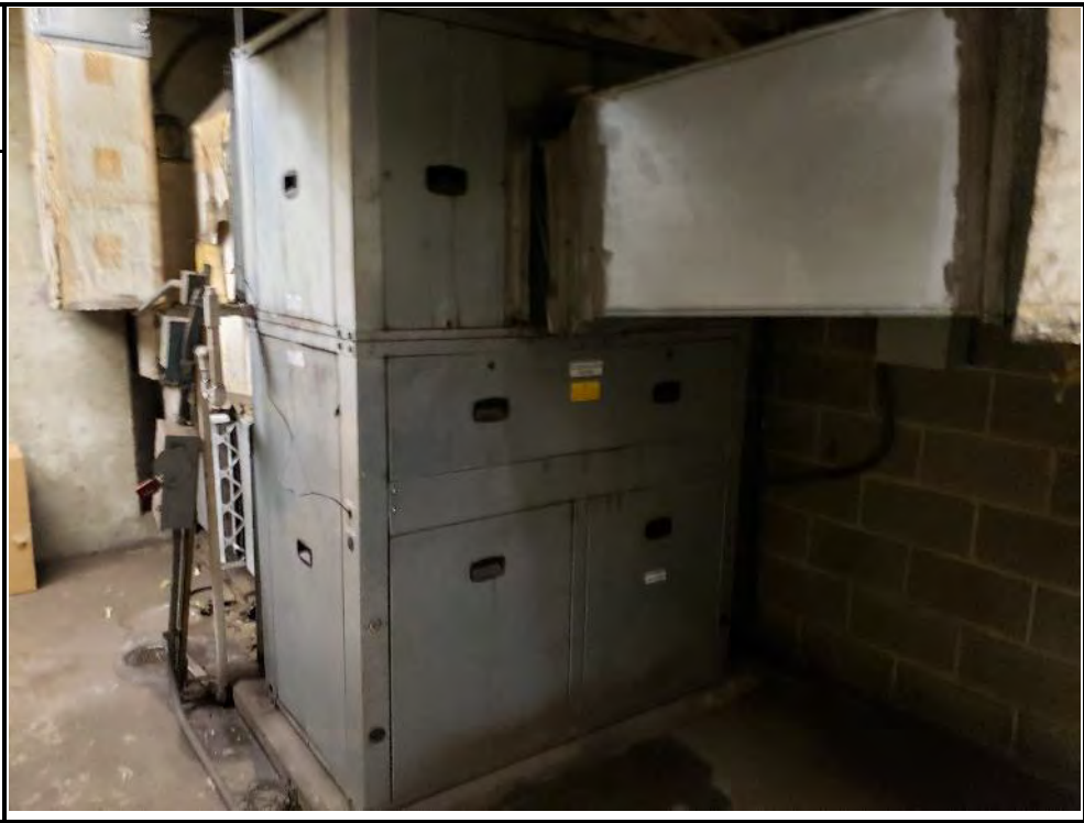
View of air handlers in the Mechanical Equipment Room in the North Service Area.
