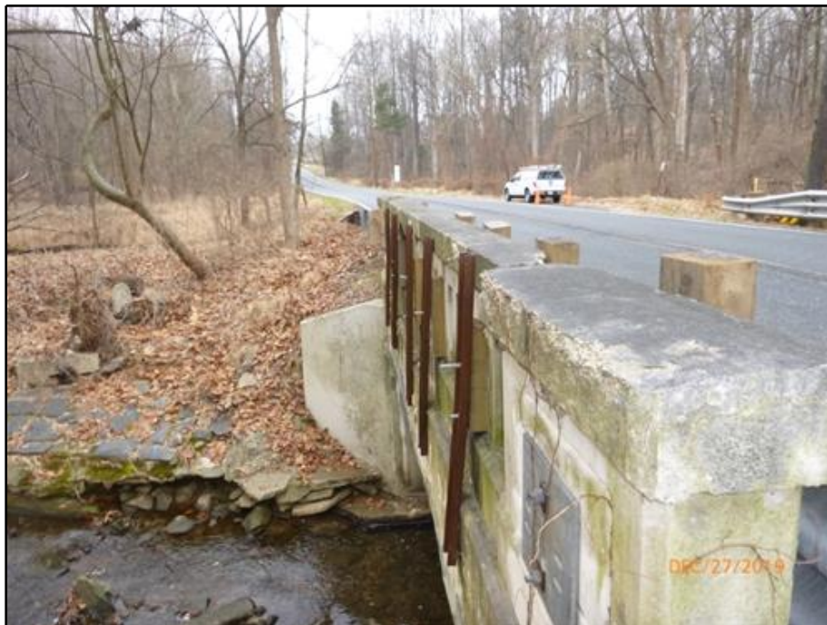
24. Back face of the newly installed three beam traffic barrier (West Traffic Barrier shown)
