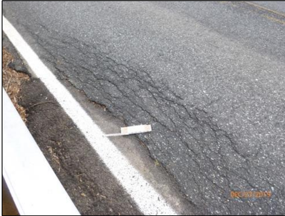
31. Map cracking at the Northwest Approach, 3' north of the bridge rail
