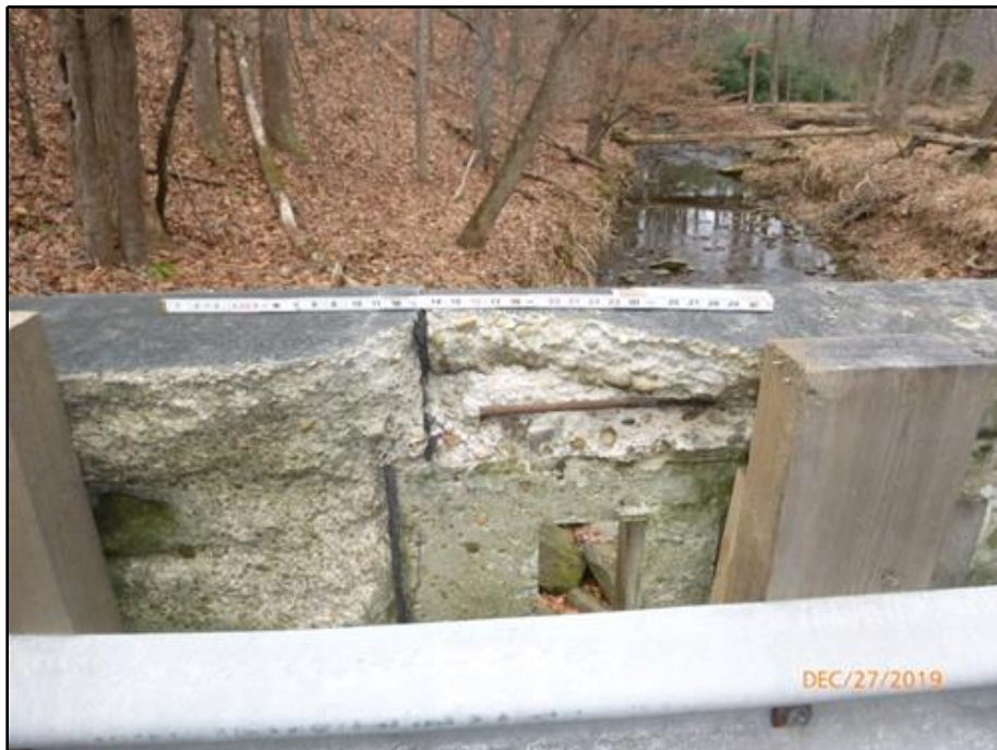
18. Spall with exposed reinforcement in the top face of the West Bridge Railing at the south end
