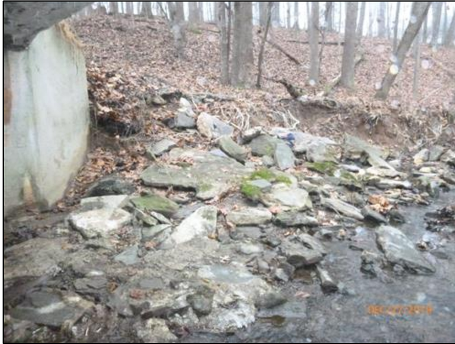
25. Southwest Slope Protection has failed due to erosion and riprap has fallen into the channel and mostly washed away
