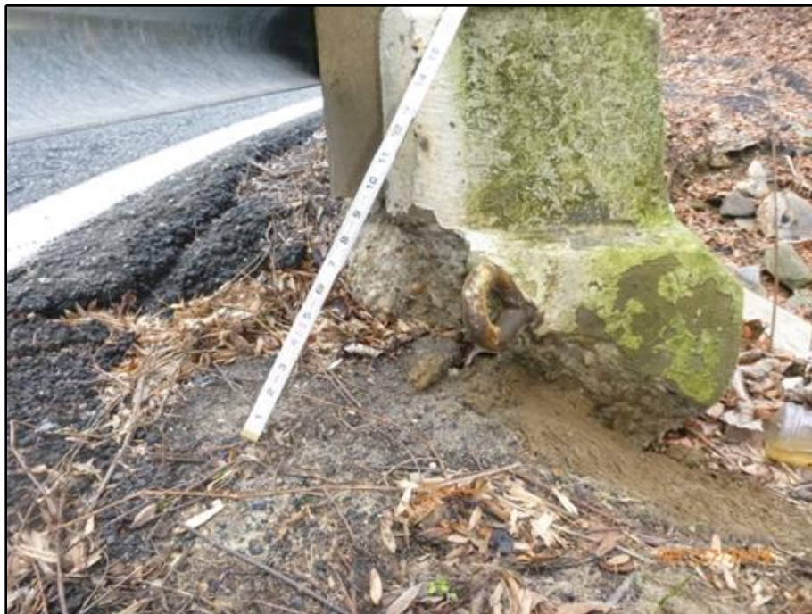
16. Spall at the base of the north end post on the West Bridge Railing
