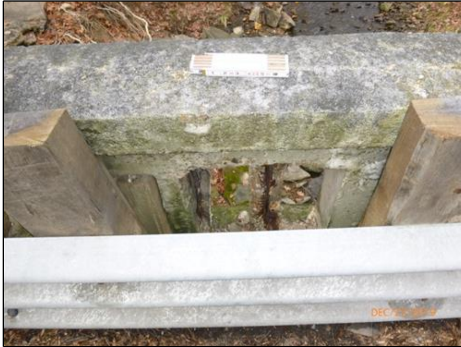
17. Balusters 10 and 11 of the West Bridge Railing are spalled with exposed reinforcement
