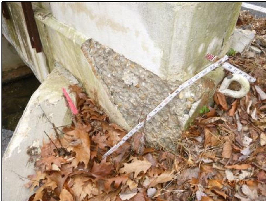
20. Spall in the base of the east face of the north end post on the East Bridge Railing
