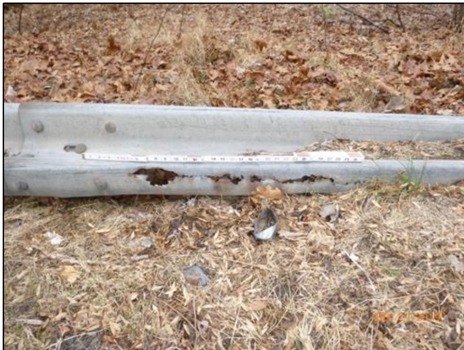
26. Section loss on the Northwest Approach Traffic Barrier between the 1st and 2nd posts from the north end
