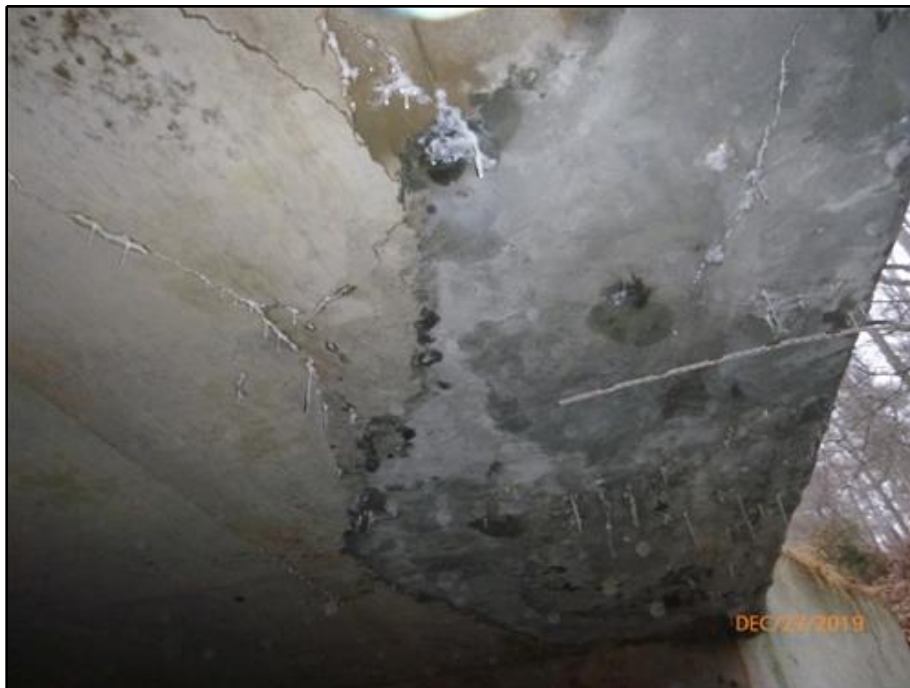
14. Hollow sounding patch in the soffit at the west edge
