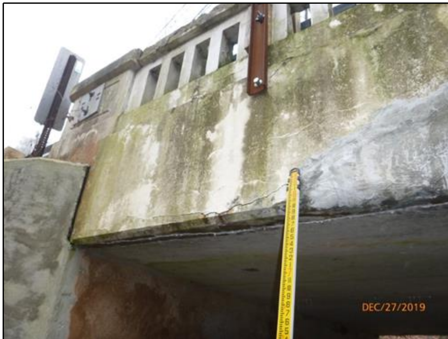
12. Delamination on the East Fascia just south of the patch
