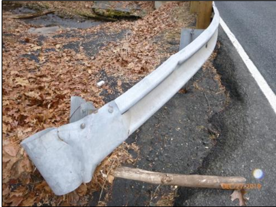
27. Impact damage to the Southwest Approach Traffic Barrier End Treatment
