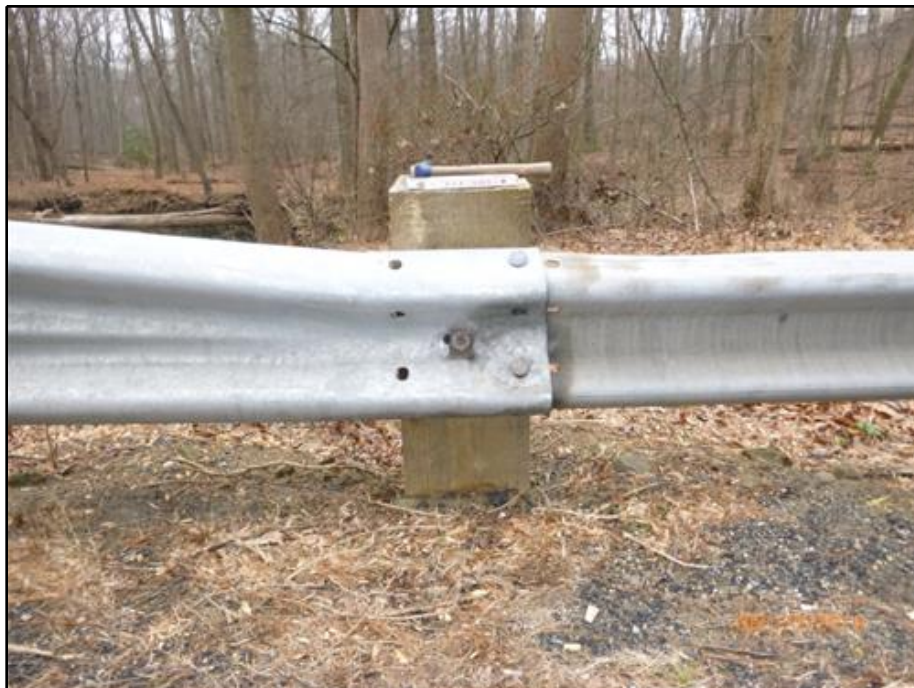
28. Missing W-beam splice bolts and the W-beam splice is lapped incorrectly at the 2nd post from the bridge for the Southeast Approach Traffic Barrier
