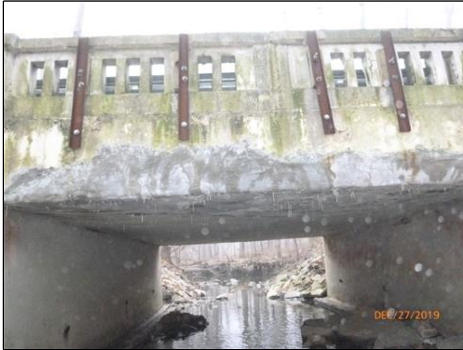
13. Hollow sounding patch on the West Fascia
