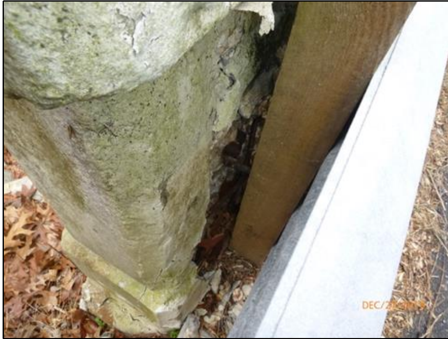
21. Spall with exposed reinforcement in the base of the west face of the East Bridge Railing, at the first traffic barrier post from the north end
