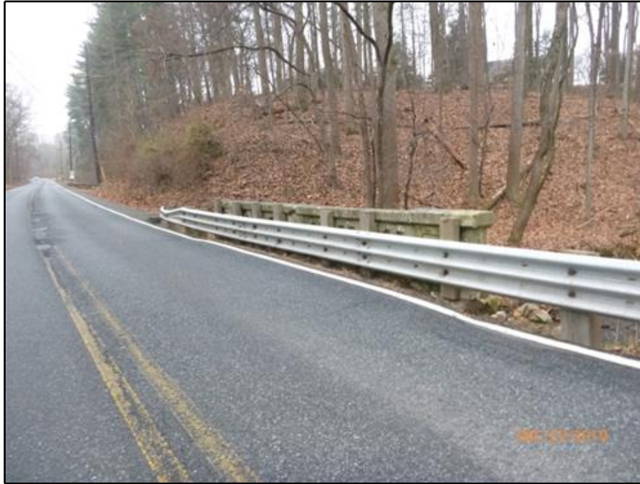
23. Front face of the newly installed three beam traffic barrier (West Traffic Barrier shown)
