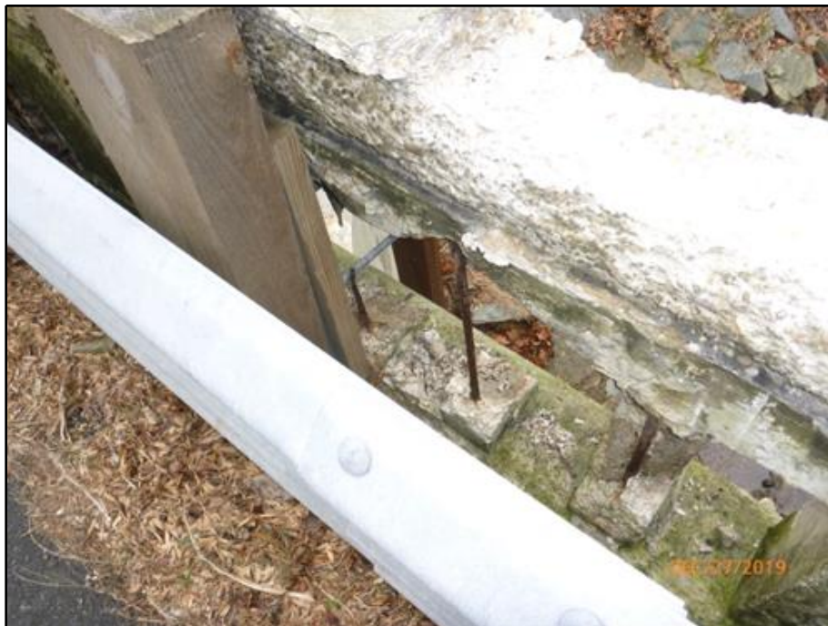
22. Balusters 1 and 2 of the East Bridge Railing are missing
