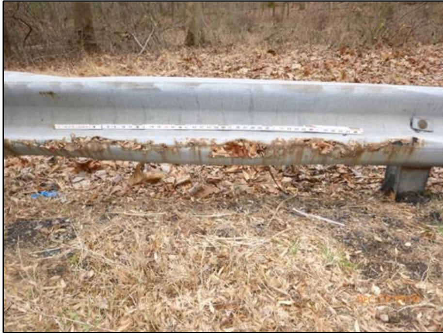
29. Section loss on the Southeast Approach Traffic Barrier between the 2nd and 3rd posts from the south end
