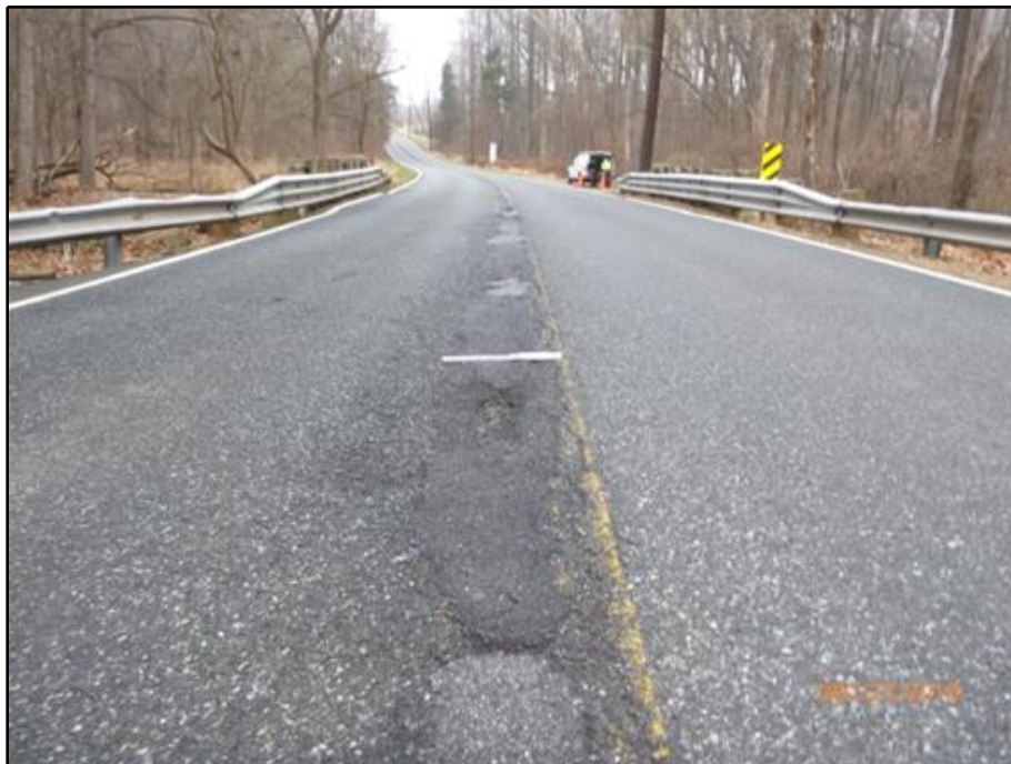
32. Potholes within the patch along the centerline of the South Approach
