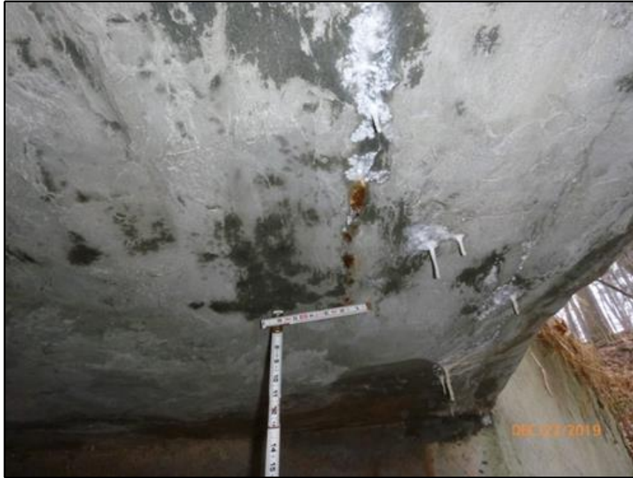
15. Exposed reinforcement in the south end of the patch in the soffit at the west edge
