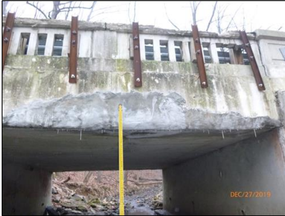
11. Hollow sounding patch on the East Fascia
