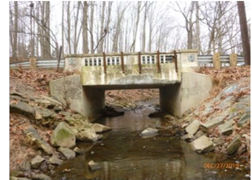
Undersized Bridge Opening
