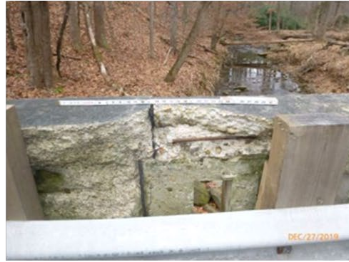
Spalled Concrete Railing
