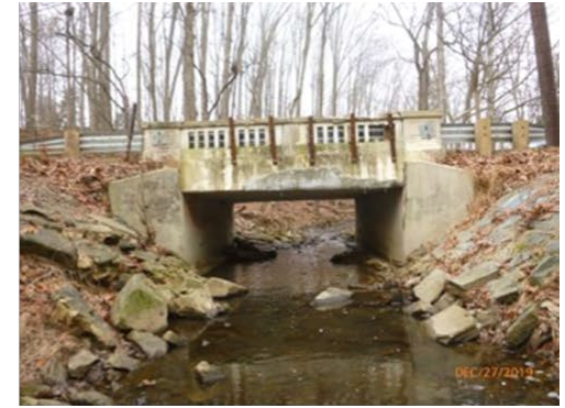
Undersized Bridge Opening
