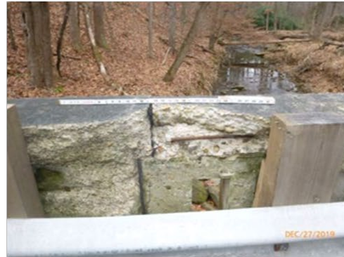
Spalled Concrete Railing
