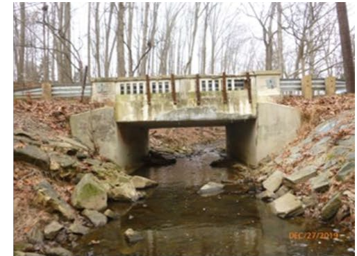
Undersized Bridge Opening
