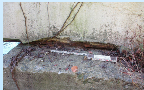
Spall at Fascia Face of Deck and Exposed at Bottom Flange of Beam
