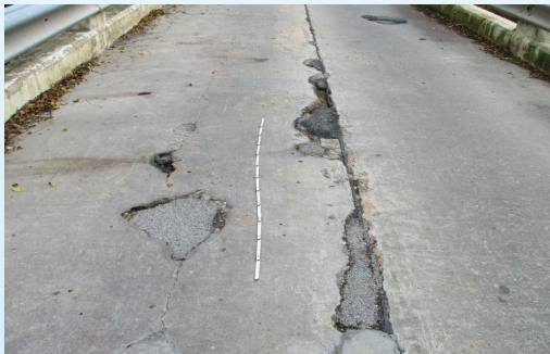
Failing Asphalt Patches
