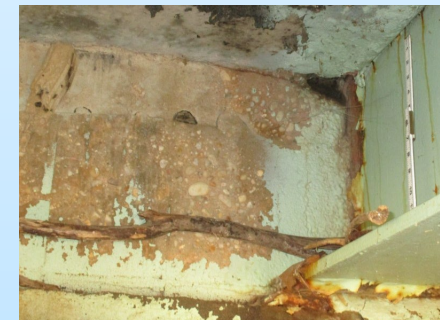
Hole at Backwall of East Abutment
