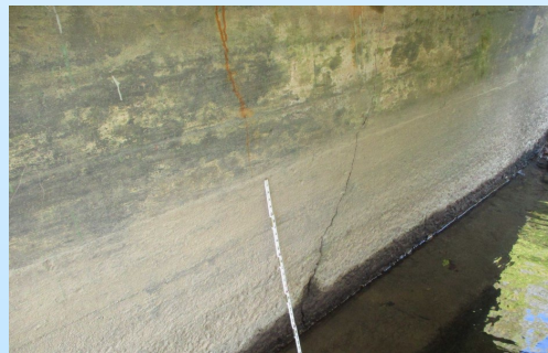
Full Height Vertical Crack at West Abutment Concrete Encasement
