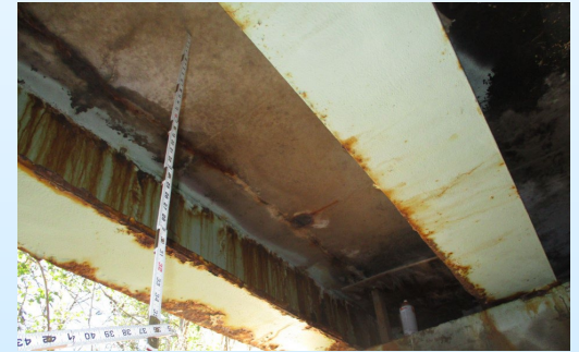
Spall underneath Deck
