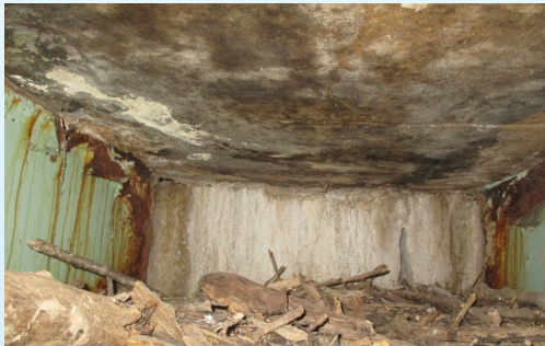
Heavy Efflorescence at Concrete Backwall of West Abutment
