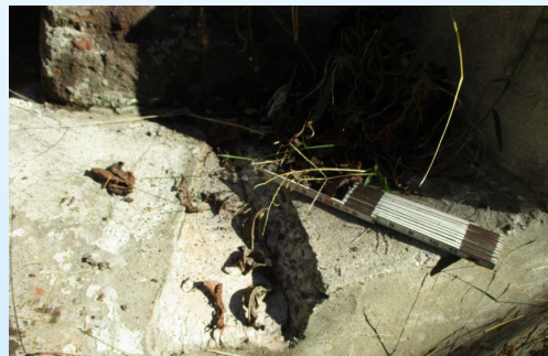
Spall at Top of East Abutment Concrete Encasement
