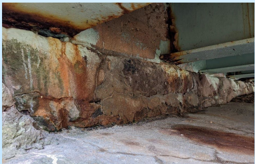
Spall at Concrete Backwall and Stone Beam Seat of East Abutment
