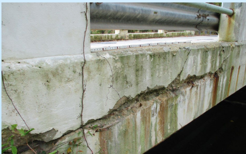
Spall at Fascia Face of Deck and Exposed at Top Flange of Beam
