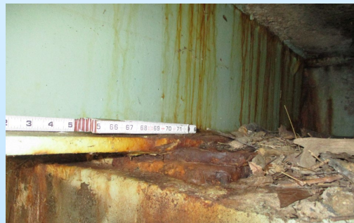
Rust and Heavy Corrosion at Bearings
