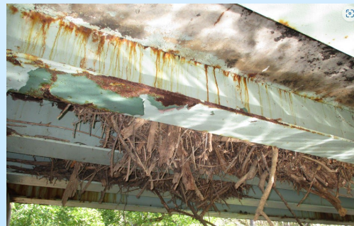
Flood Debris Caught between Beams
