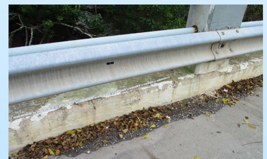
Spall at Curb
