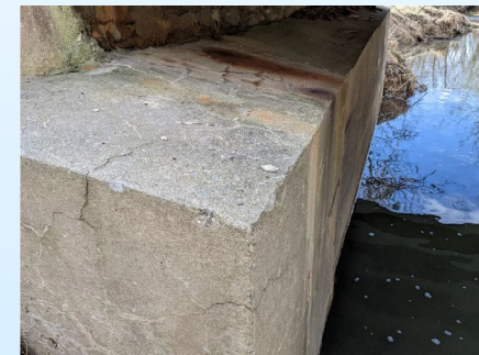
Crack at Top of East Abutment Concrete Encasement
