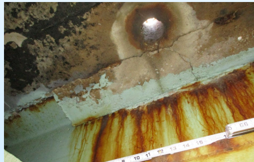
Spall underneath Deck
