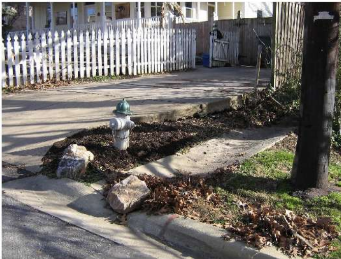
Photo 11 – Concrete Swale at 5123 Waukesha
