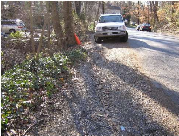
Photo 8 – Eroded Ditch on Tuscarawas Road
