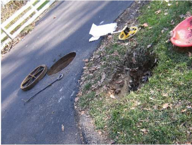
Photo 5 – Converted Inlet at 5317 Tuscarawas
