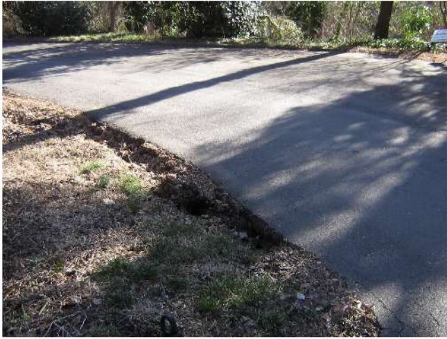
Photo 13 – Soil Erosion Along Edge of Alexander Road
