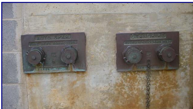
Adjacent, but Separate Sprinkler and Standpipe Connections
