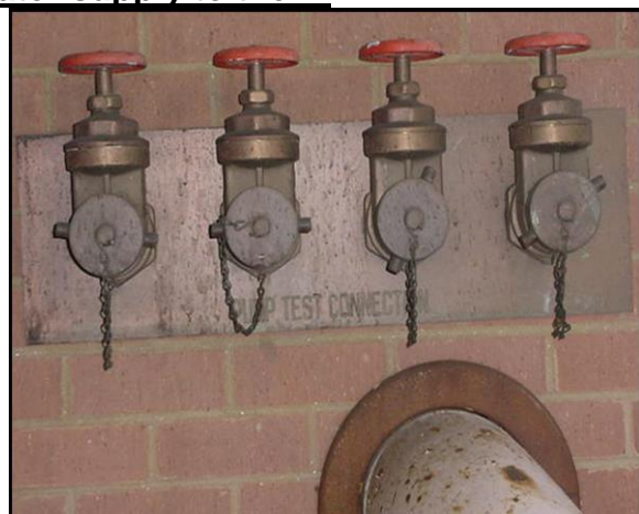
Fire Pump Test Header
