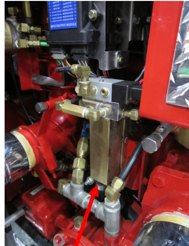
Primer located behind curbside pump panel
