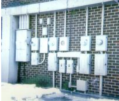
Commercial meter bank showing main disconnect, meters and individual occupancy disconnects.
