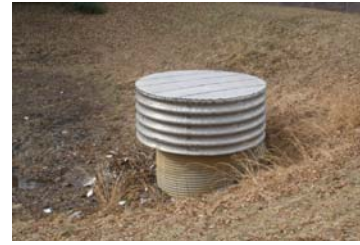
FIGURE 3. EXISTING RISER (POND CONTROL STRUCTURE) TO BE REPLACED WITH A 10' X 20' CAST-IN-PLACE REINFORCED CONCRETE RISER W/ TRASH RACK AND MANHOLE COVER.
