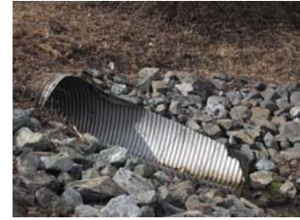
FIGURE 4. EXISTING INFLOW PIPE TO BE MODIFIED. DAYLIGHTED SEGMENT TO BE REMOVED AND A NEW CONCRETE HEADWALL TO BE INSTALLED AT END OF PIPE.
