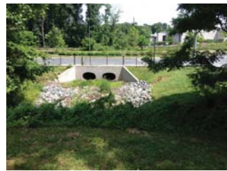
FIGURE 5. PROPOSED RETROFIT WILL HAVE MINIMAL IMPACT ON THE STILLING BASIN AND NO IMPACT ON CULVERT SYSTEM BENEATH MONTROSE PARKWAY.
