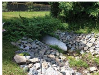
FIGURE 6. EXISTING OUTFALL PIPE TO BE MODIFIED. DAYLIGHTED SEGMENT TO BE REMOVED AND EXISTING PIPE TO BE SLIP-LINED WITH 54\"/>
